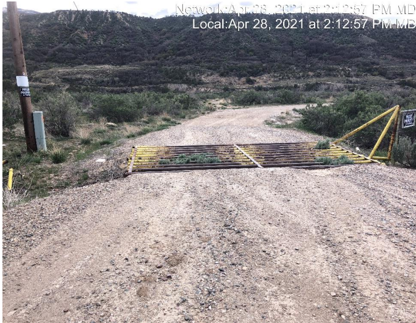
Photo #3661 Tracking control at entrance to location insufficient.
