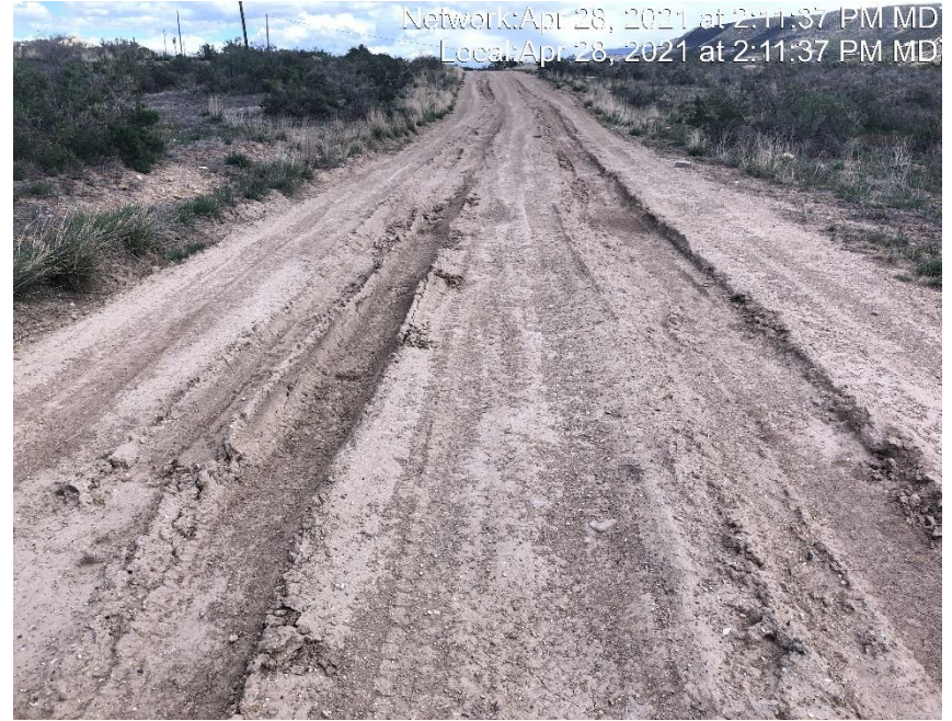
Photo #3660 Access road lacks stabilization.
