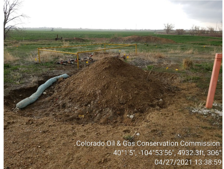
Inadequate fencing & storm water BMPs
