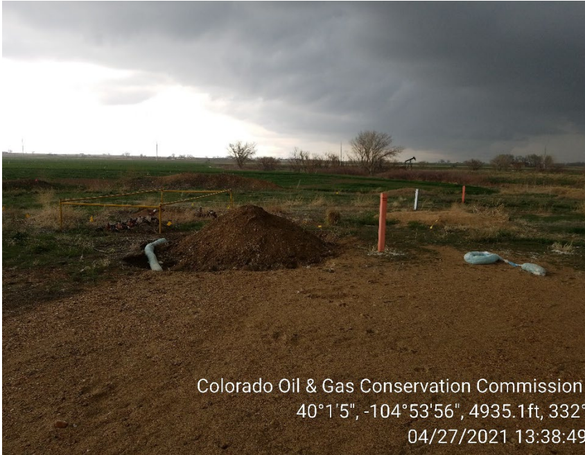
Inadequate fencing & storm water BMPs
