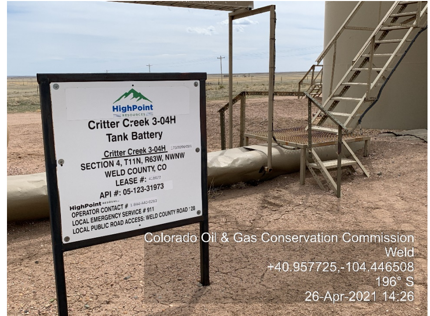
Photo #4 Critter Creek 3-04H Battery site Active Battery sign
