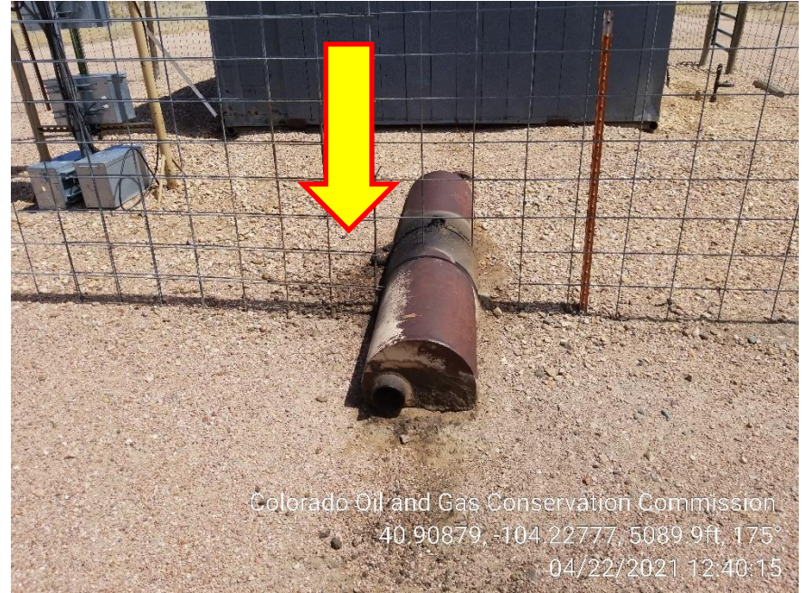
Photo 4 – Stained Soil at Exhaust
