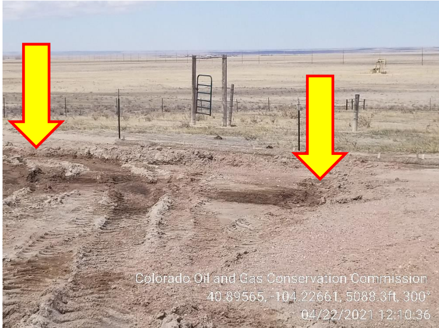
Photo 7 – Storm Water erosion
