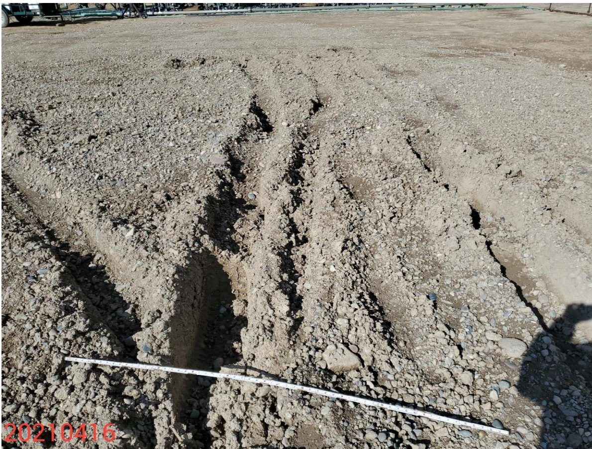
Photo 1: Photo taken from the Location. Photo shows control measures to stabilize/protect unpaved areas of the Location remain missing or insufficient. 6 foot measuring stick for reference.
