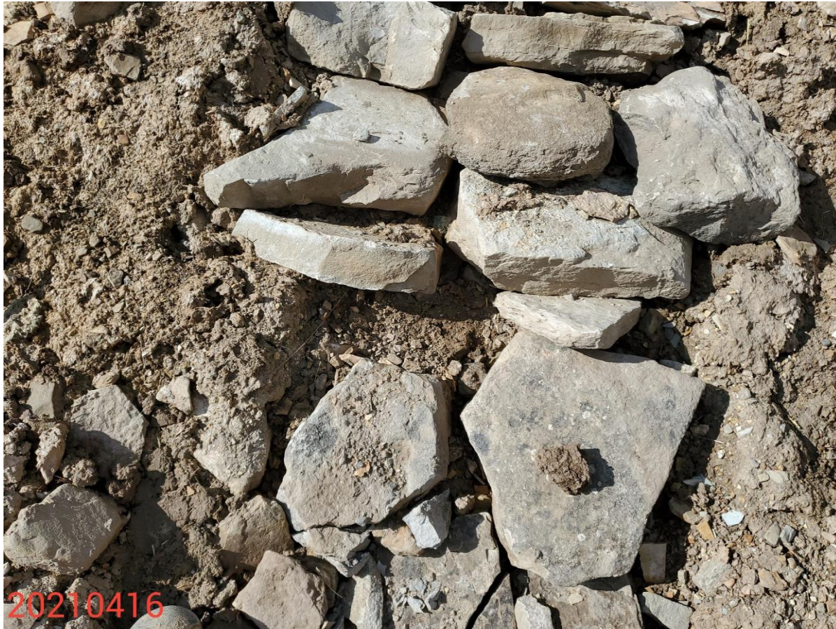
Photo 5: Continued from photo 4. Photo shows control measure has not been installed in accordance with good engineering practices; BMP insufficient to stabilize slopes.
