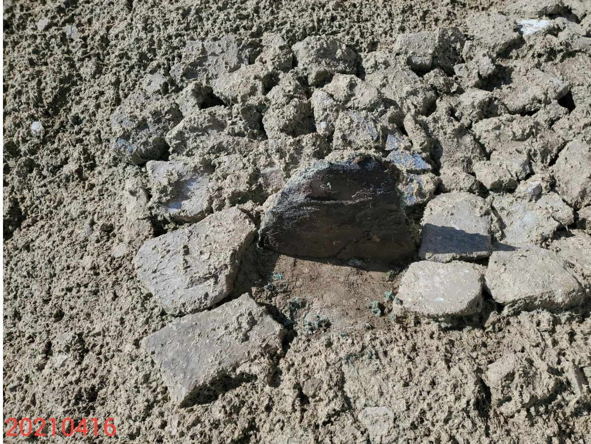
Photo 28: Continued from photo 27. Photo shows Operator has implemented sediment traps along the access road; control measures have not been installed with a geotextile liner in accordance with good engineering practices.
