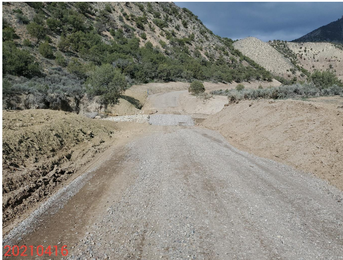
Photo 26: Photo taken from the stream crossing along the access road. Photo shows additional work has been performed at the stream crossing; it is unclear if work conducted will provide long term stabilization to the channel, however, control measures to prevent sediment/pollutant discharge from vehicles and equipment traveling through the intermittent stream and drainage remain missing or insufficient.
