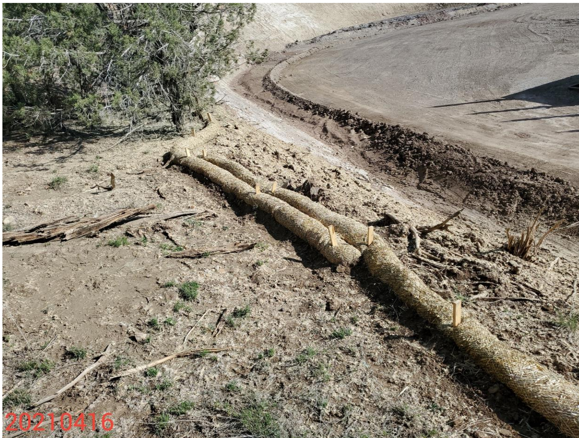
Photo 12: Photo taken from the cut slope on the west end of the Location. Photo shows area where terrace grading has been installed to address erosion concerns on the cut slope.
