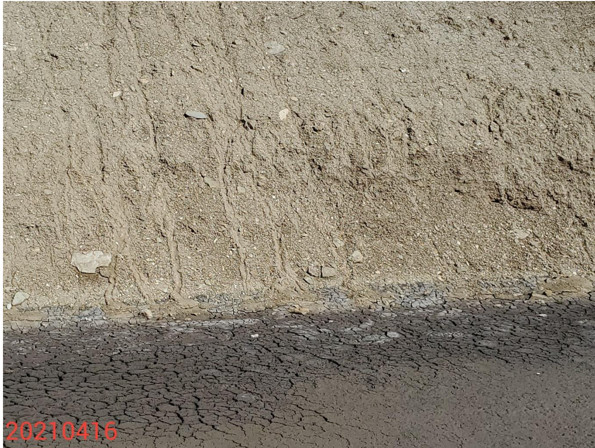
Photo 23: Continued from photo 22. Photo shows sediment deposition due to erosion at the cut slopes.
