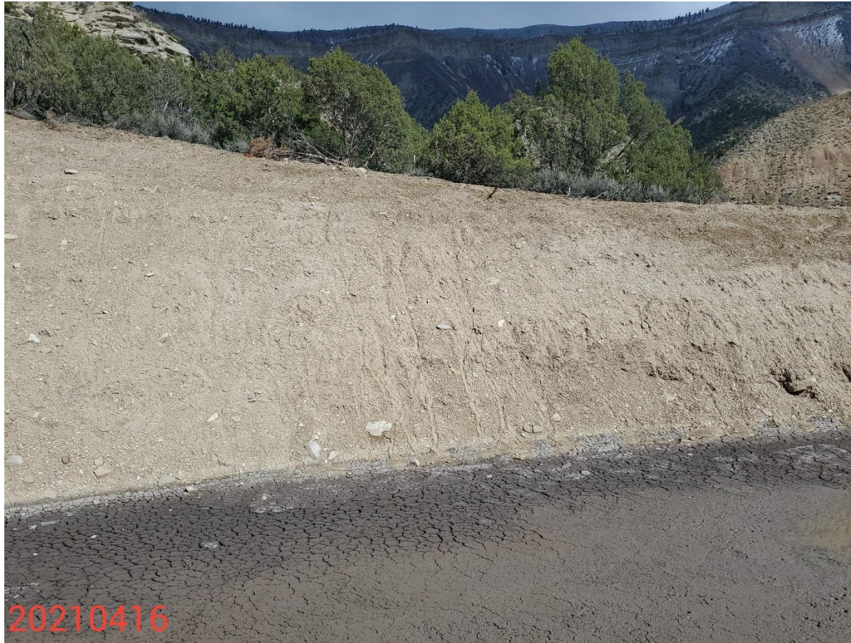
Photo 22: Photo taken from the cut slope on the north end of the Location. Photo shows rill erosion; control measures to stabilize and protect slopes of the Location, and manage runoff remain missing or insufficient.
