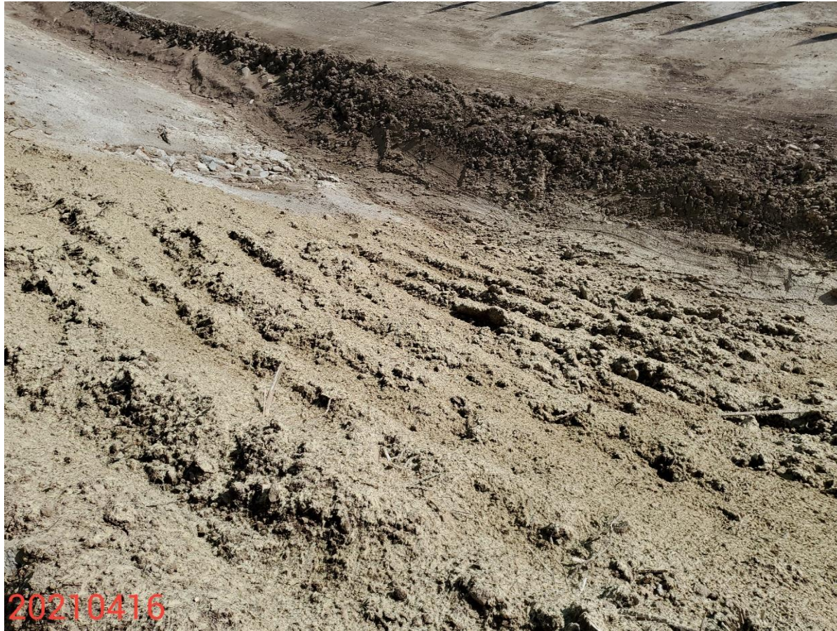
Photo 14: Photo taken from the cut slope on the west end of the Location. Photo shows area where terrace grading has been installed to address erosion concerns on the cut slope. Though hydromulch has been used in conjunction with terracing, soils remain insufficiently stabilized and protected.
