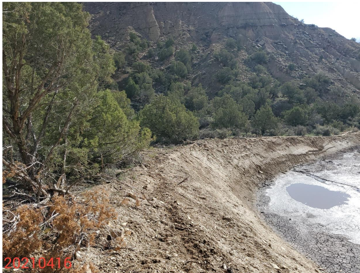
Photo 19: Photo taken from above the cut slope on the west end of the Location. Photo shows example of areas where runon control measures have not been installed; runon control measures remain missing or insufficient on the Location.
