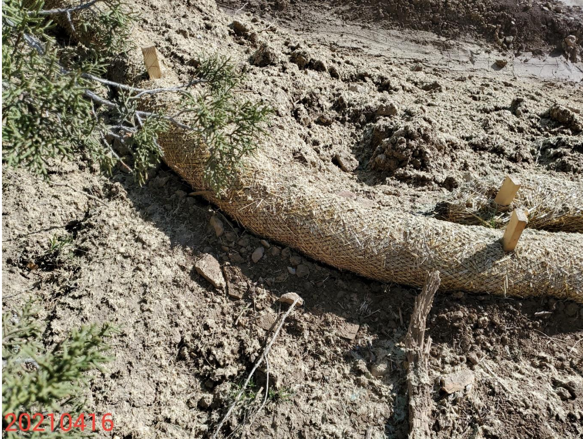
Photo 13: Continued from photo 12. Photo also shows areas of erosion logs that do not appear to have been properly backfilled to prevent water movement under the control measure.
