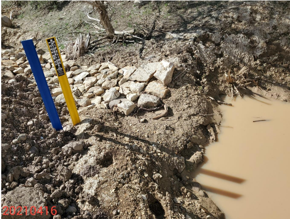
Photo 3: Photo shows sediment trap on the southwest end o the Location. Outlet at trap has not been installed in accordance with good engineering practices.
