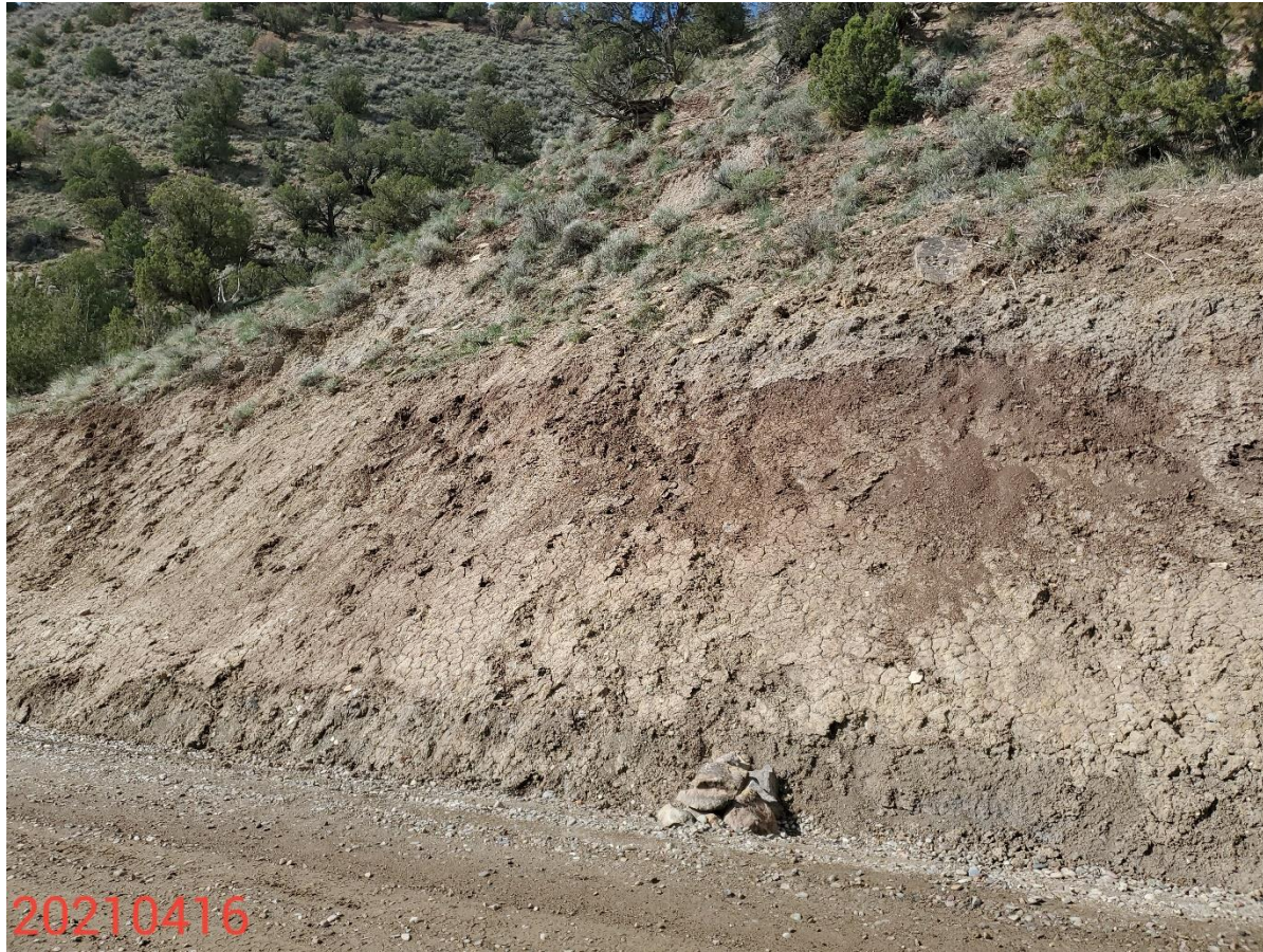
Photo 24: Photo taken from the access road. Photo shows control measures to stabilize/protect slopes remain missing or insufficient.
