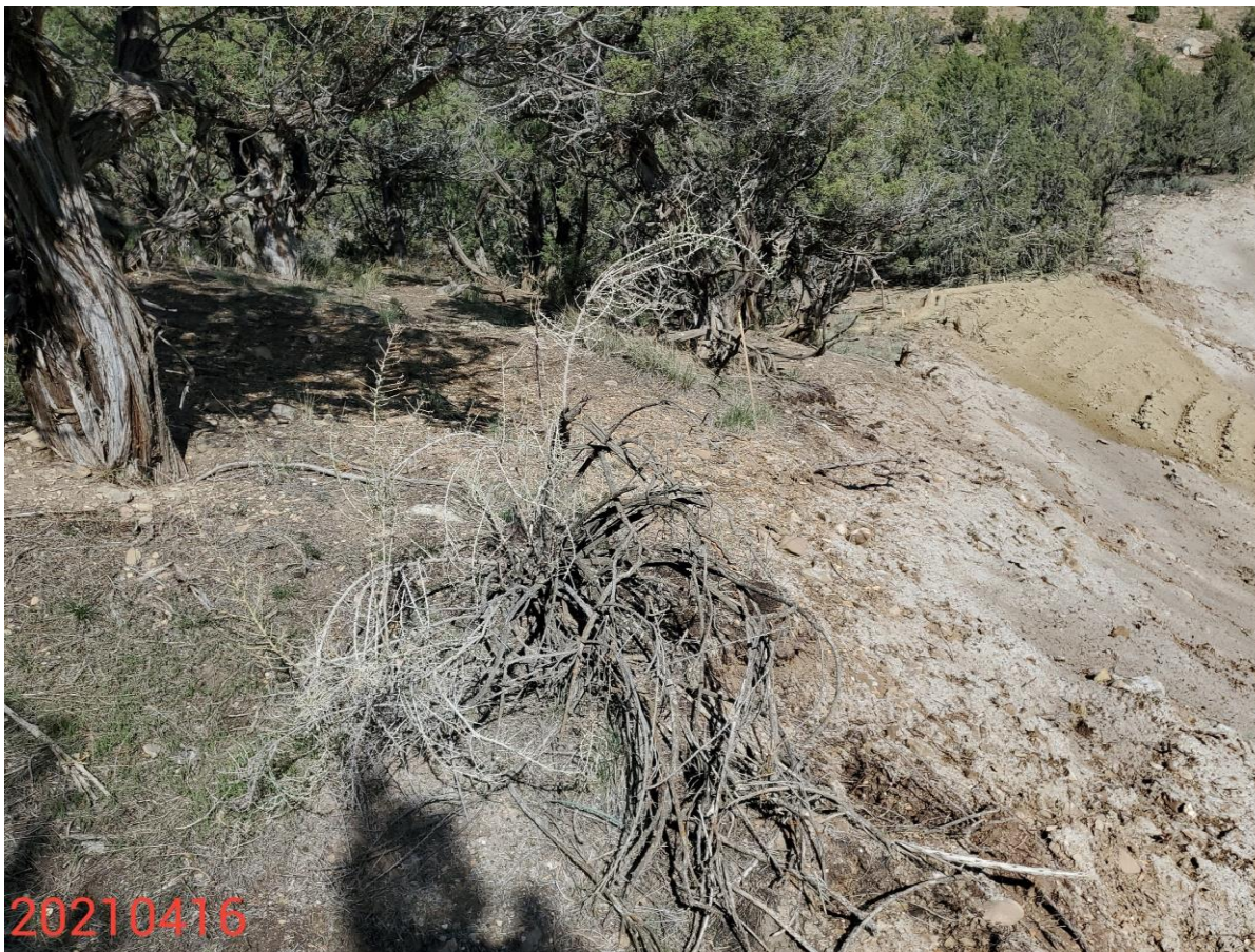
Photo 11: Photo taken from above the cut slope on the west end of the Location. Photo shows example of areas where runon control measures have not been installed; runon control measures remain missing or insufficient on the Location.
