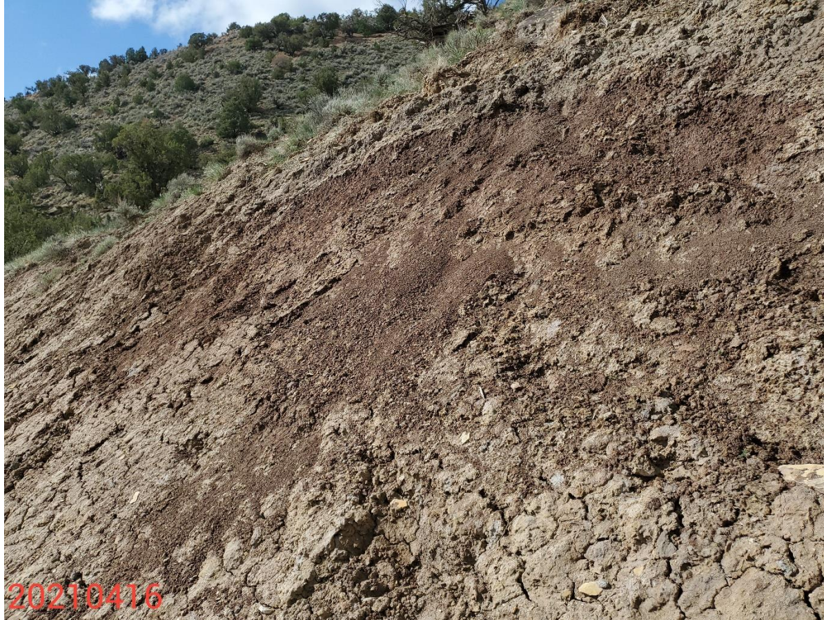
Photo 25: Photo taken from the access road. Photo shows control measures to stabilize/protect slopes remain missing or insufficient.
