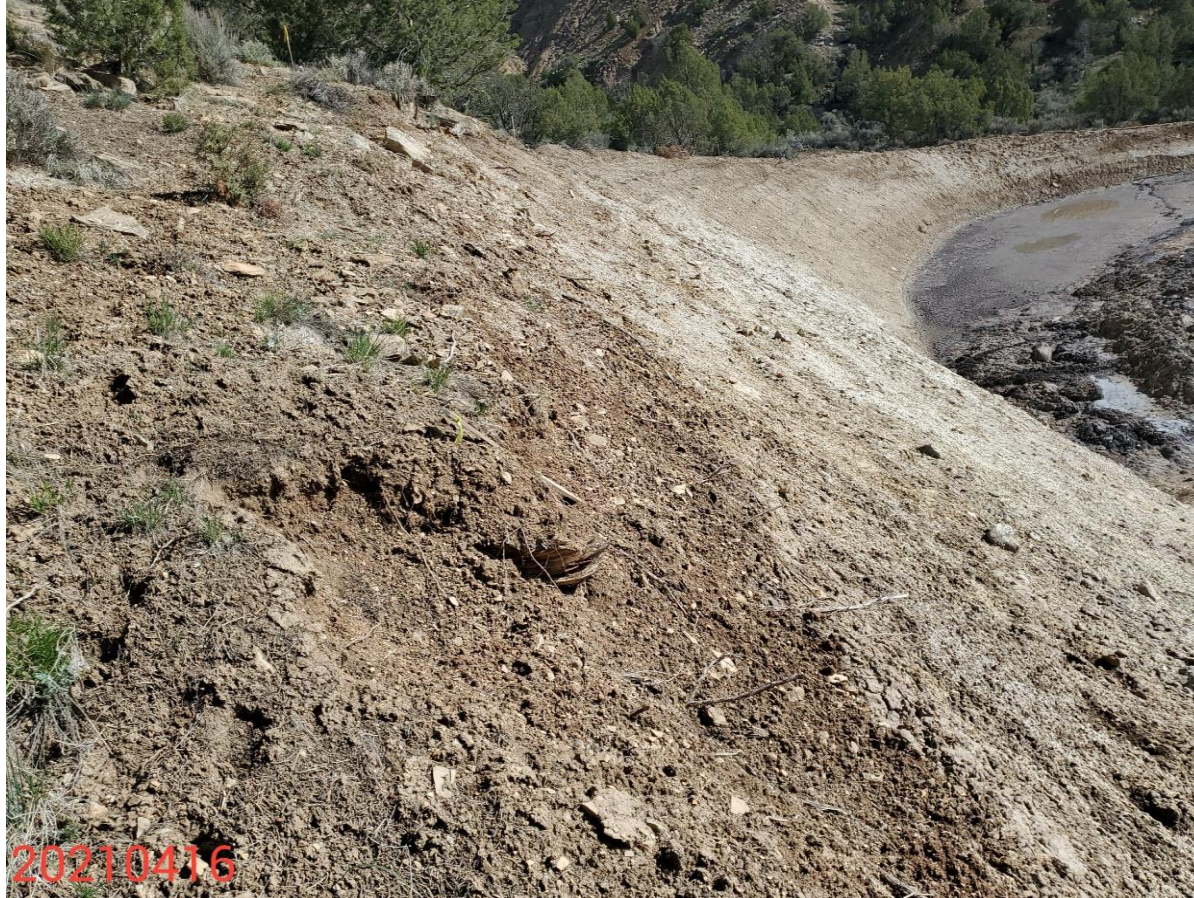
Photo 18: Photo taken from above the cut slope on the west end of the Location. Photo shows example of areas where runon control measures have not been installed; runon control measures remain missing or insufficient on the Location.
