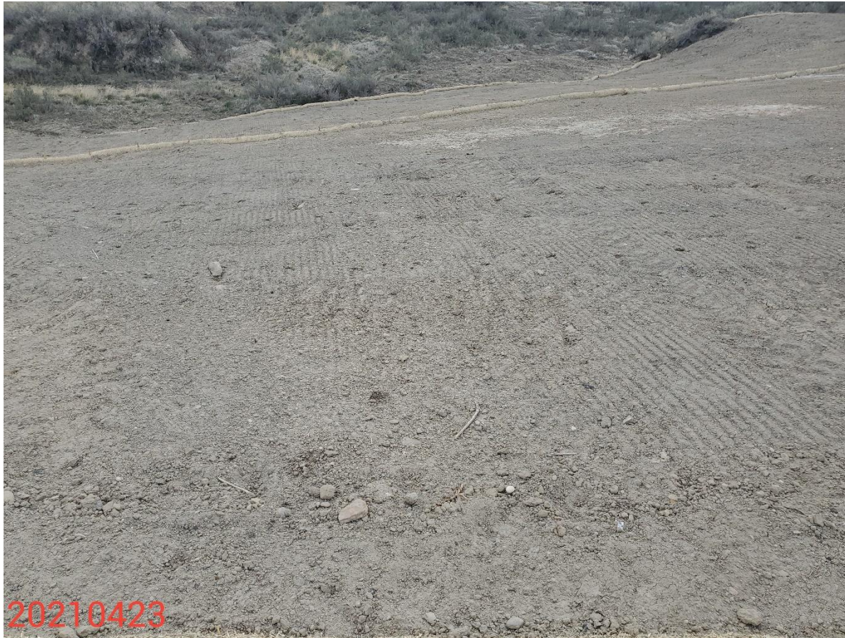
Photo 2: Photo taken from the east end of the Location, facing east. Photo shows additional erosion logs have been installed. Unclear if BMPs are sufficient or adequate for the site's conditions
