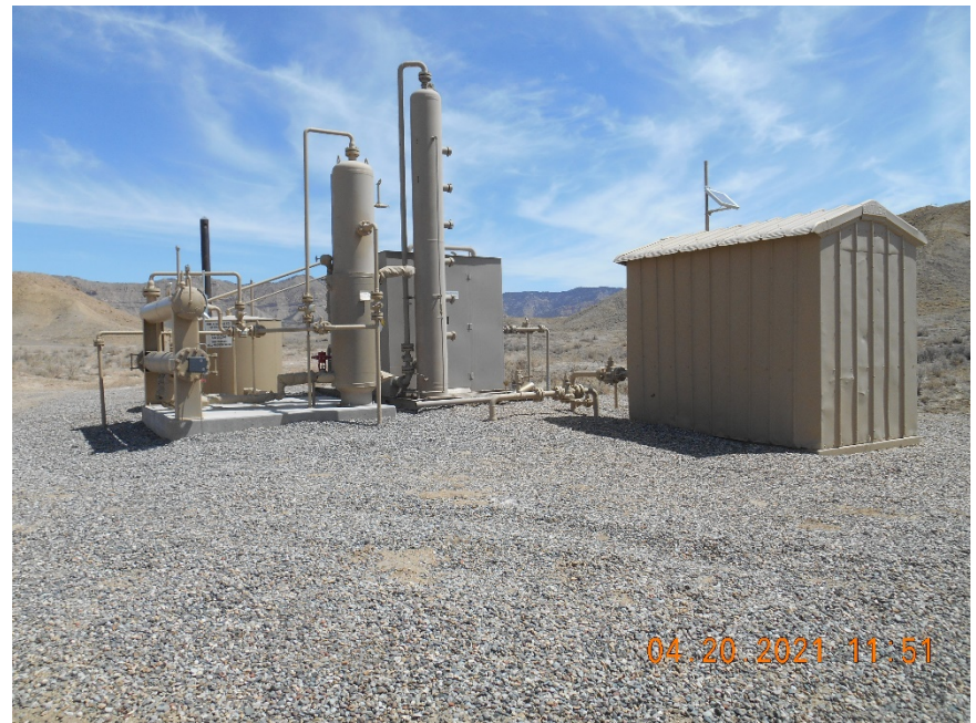
Separator, Dehydrator, Meter housing and Tank
