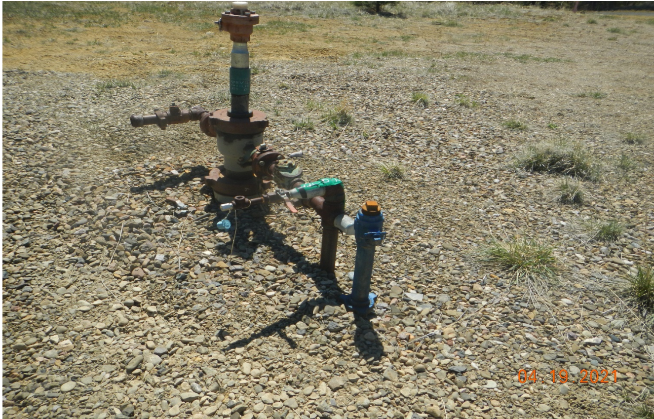
Photo 5. Risers have been locked out.
