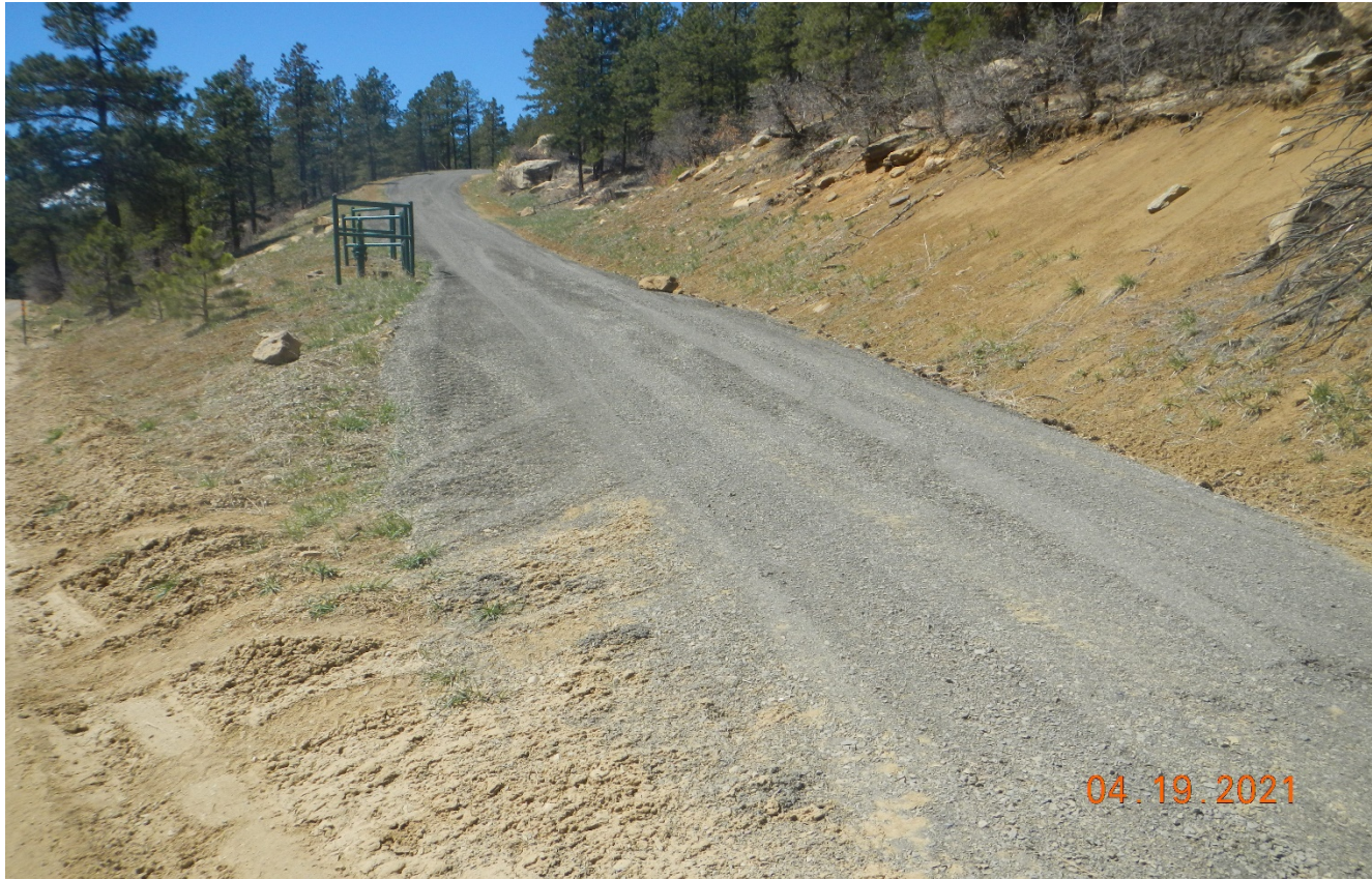
Photo 1. Facing toward the access road. Areas of erosion have been repaired and gravel was applied to the road.
