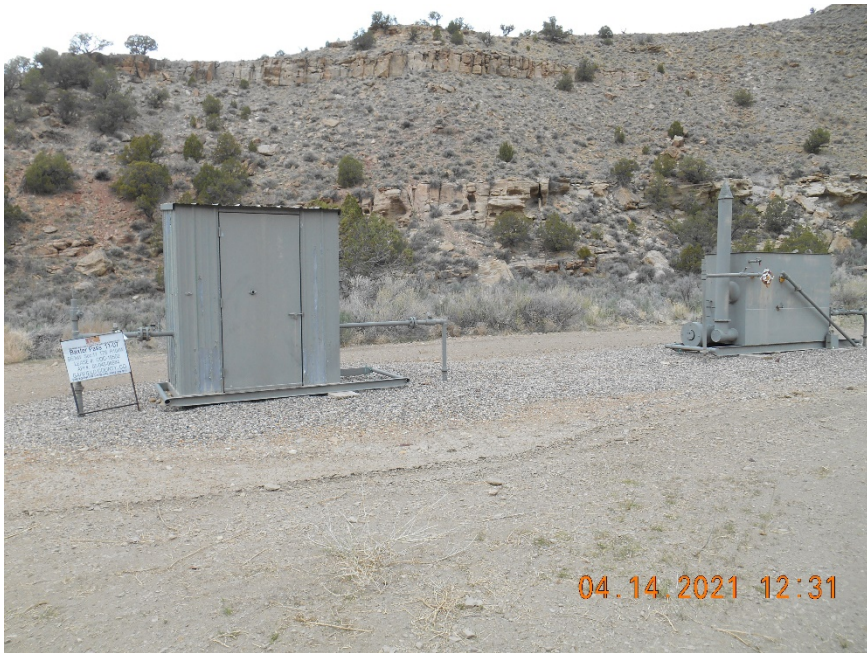
Separator and Meter housing with sign.
