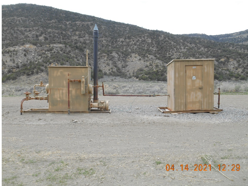
Separator and Meter housing.
