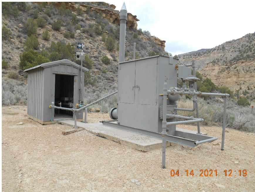
Separator and Meter housing.
