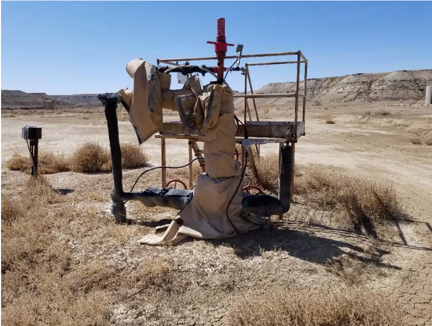
Photo 2. No bradenhead access apparent. Dried annual weeds on location.
