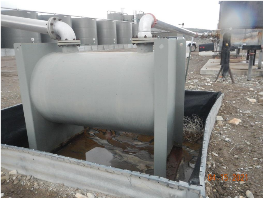
Photo#3: Equipment cellar referenced in Inspection. Note Debris weeds blown into equipment.
