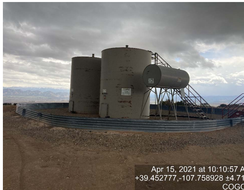
location/lack of signage
