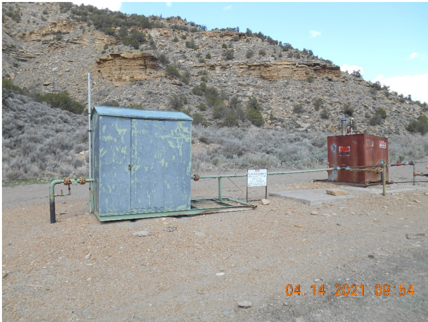
Separator and Meter Housing with sign
