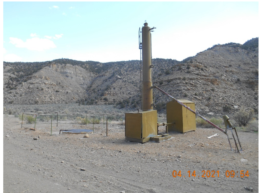
Dehydrator, Meter housing with blowdown tank.
