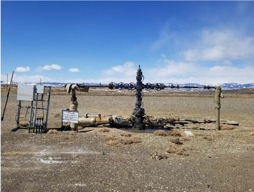
Photo 3. Wellhead locked out in TA status.
