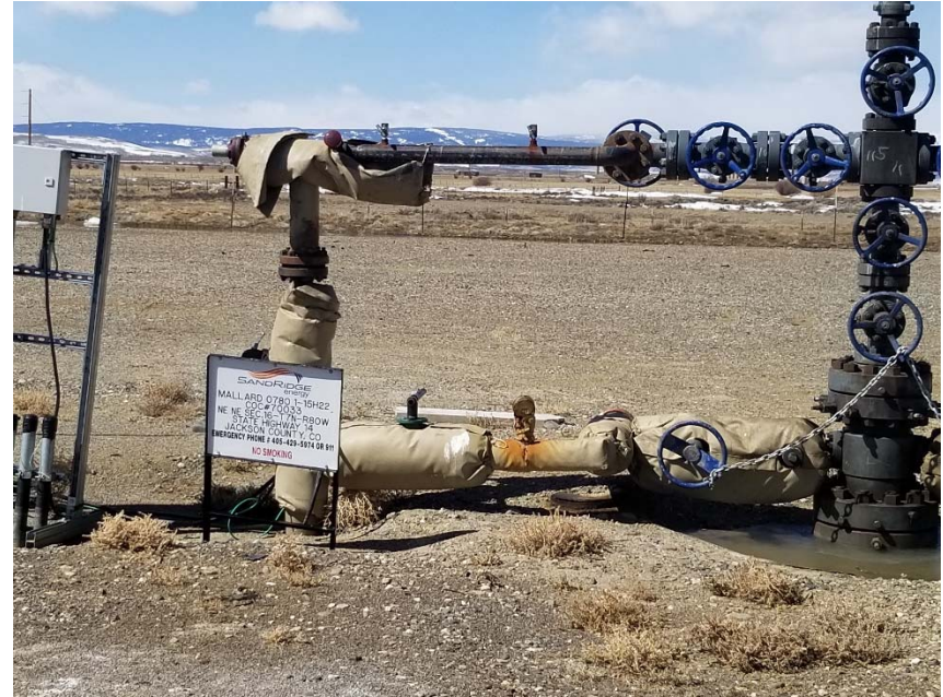
Photo 4. Wellhead sign with no updated information or emergency contact number.
