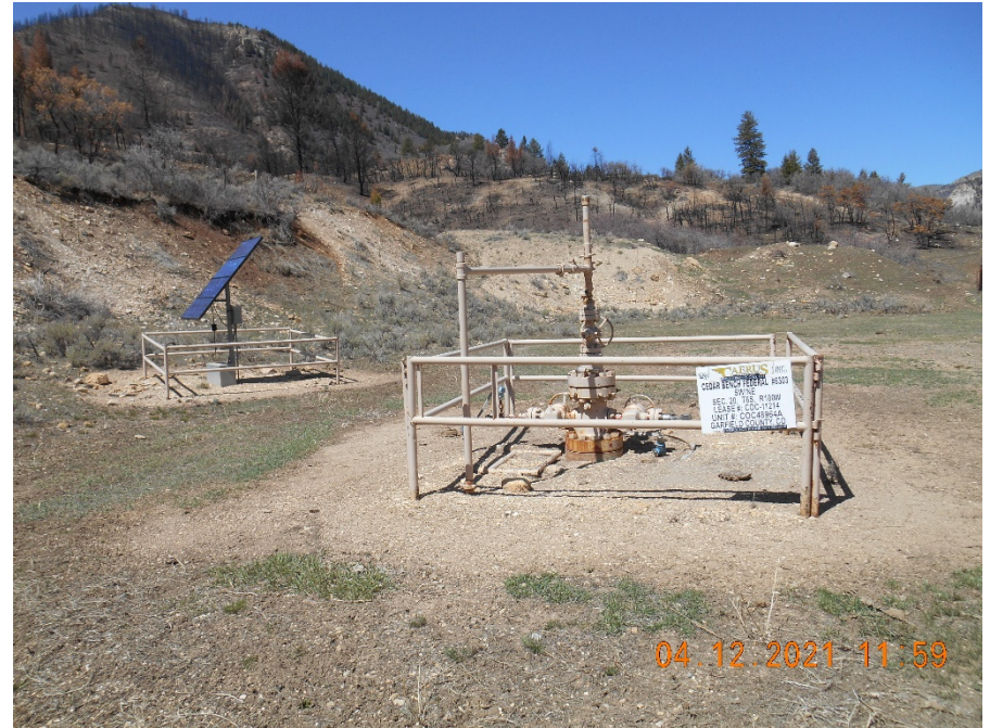
Wellhead with fence and sign
