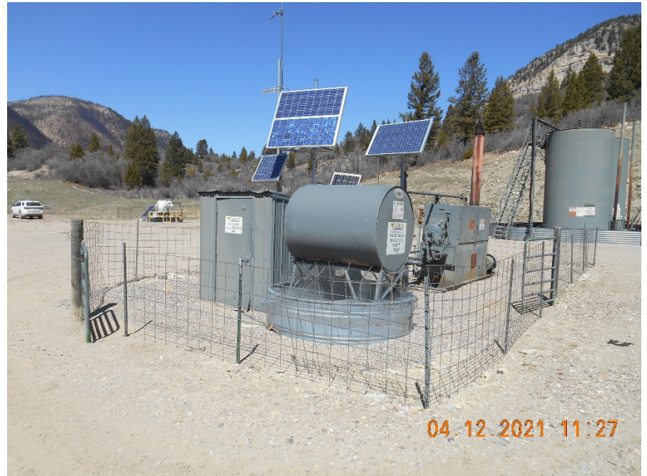
Separator and Meter housing
