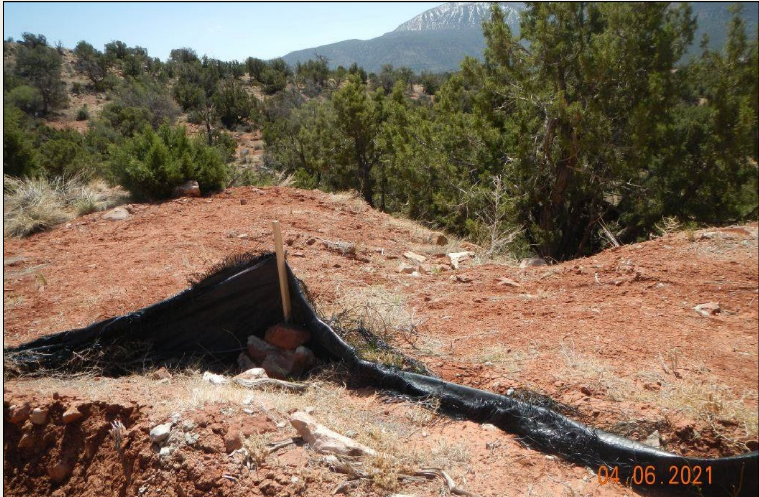
Photo 3. View of silt fence in the southeastern project area, in disrepair.
