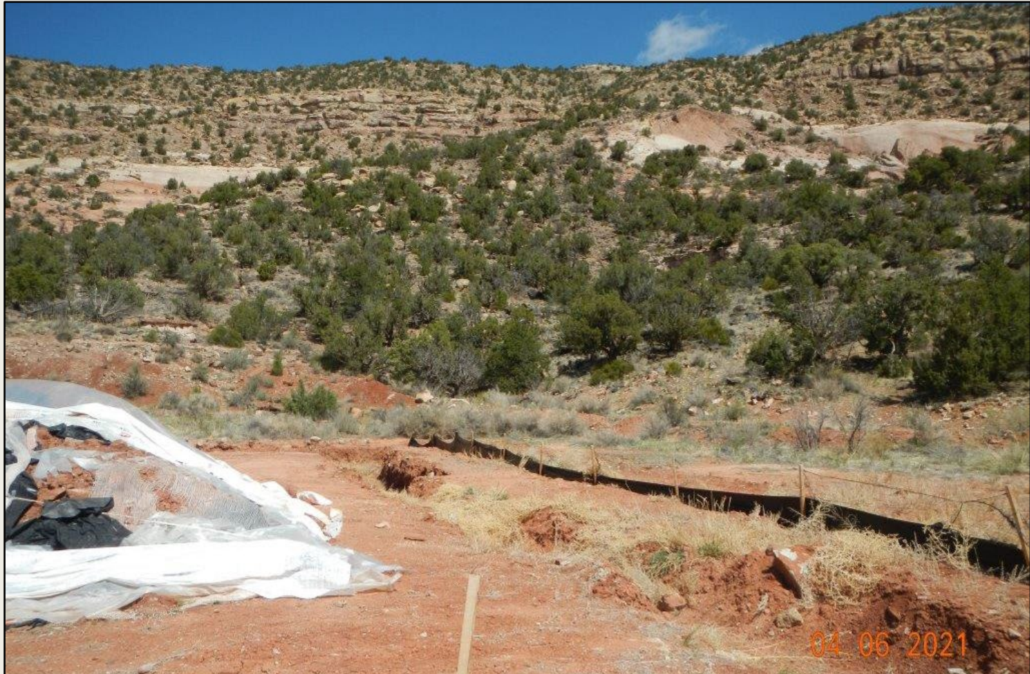
Photo 2. View of trench, approximately 2.5 feet deep and 3 feet wide, and silt fence in the eastern project area.
