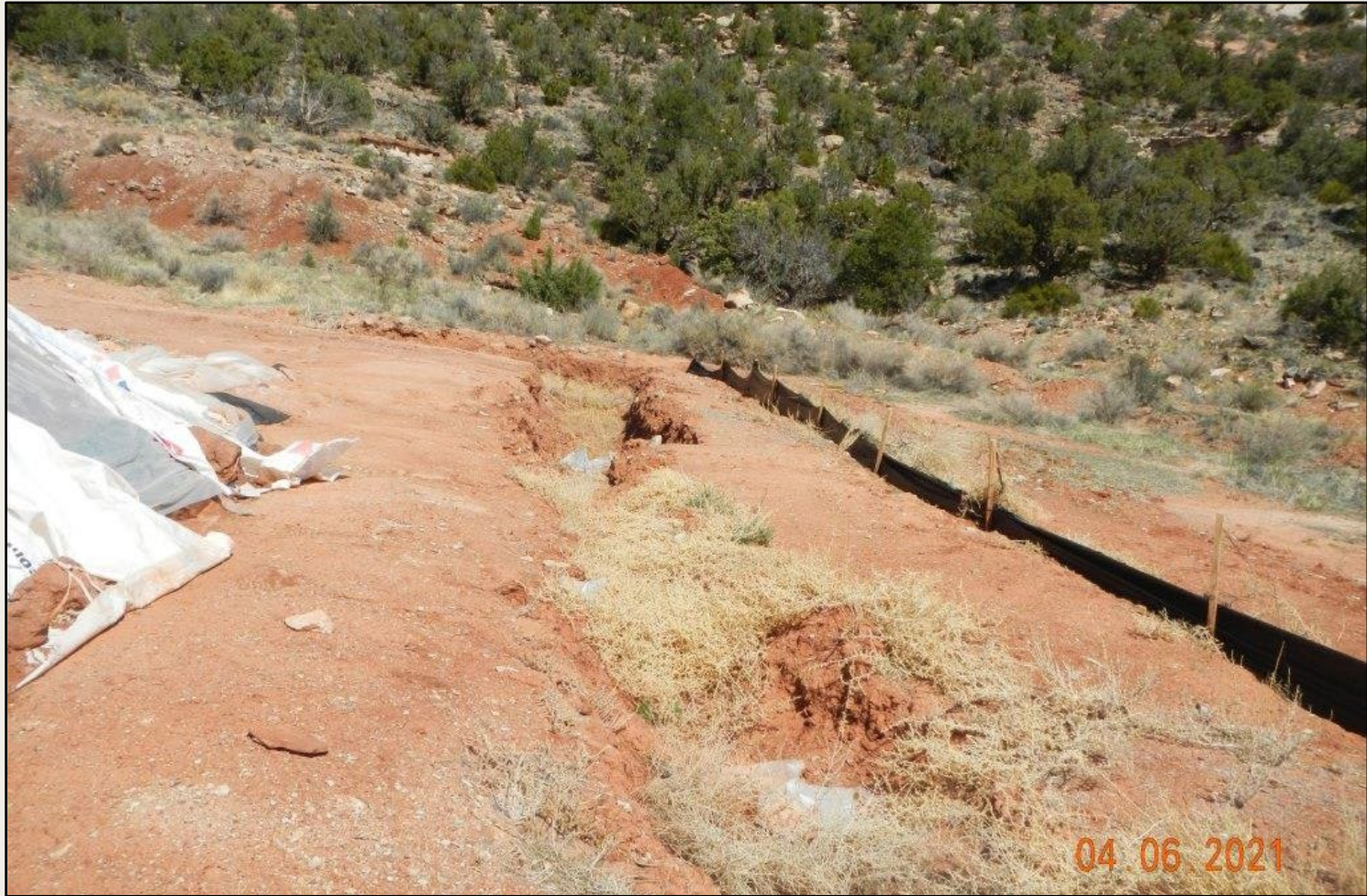
Photo 4. Another view of trench and silt fence in the eastern project area. Russian thistle and plastic debris observed in trench.
