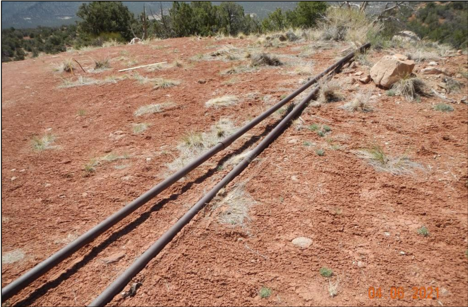
Photo 10. View of surface flowlines need to be properly abandoned.
