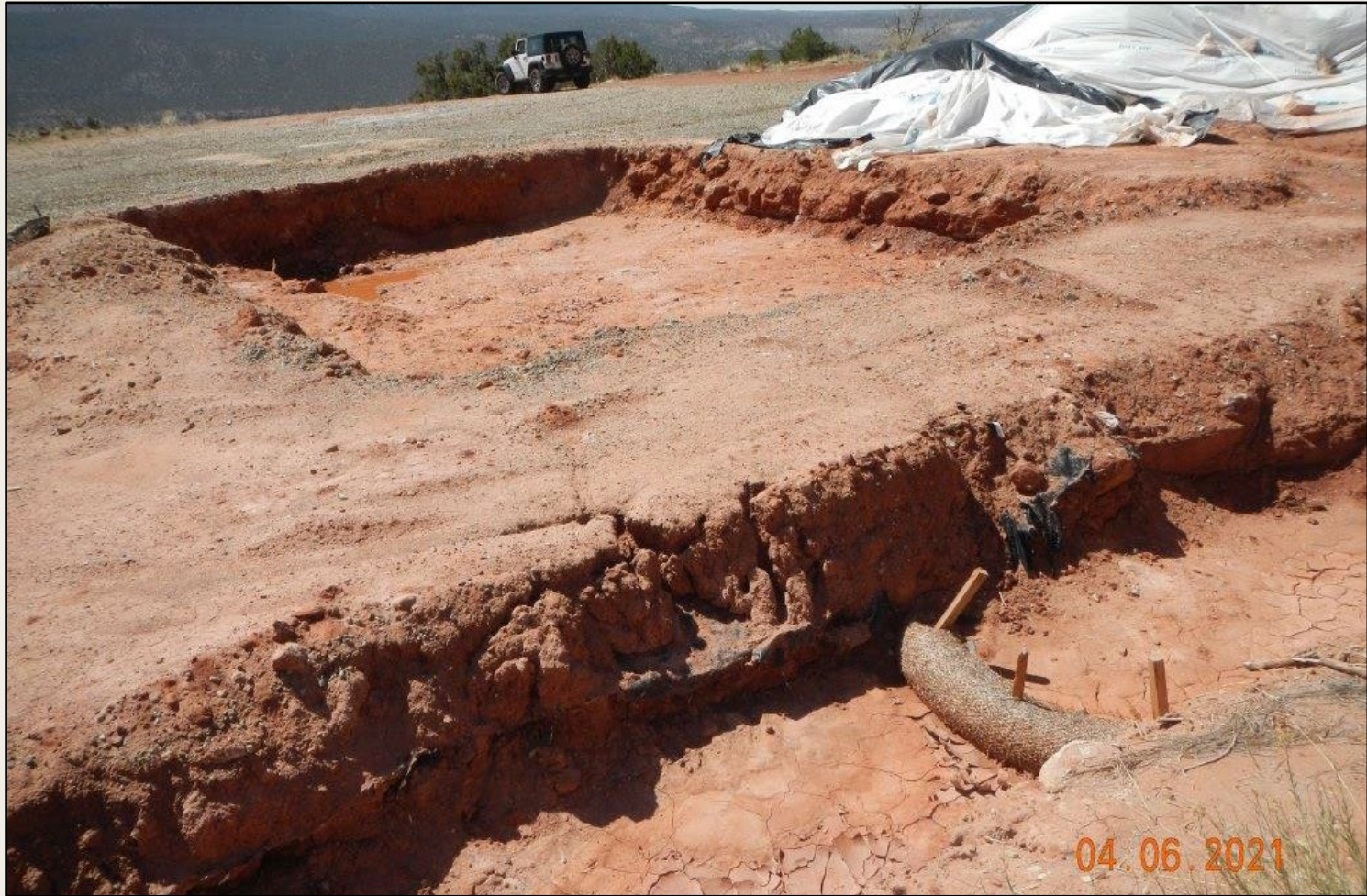
Photo 8. View of excavated area in the northern project area and trench in foreground
