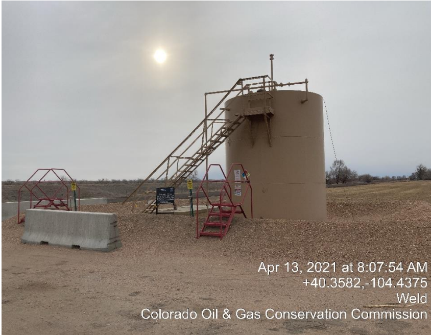
Photo #5 Tank Battery
