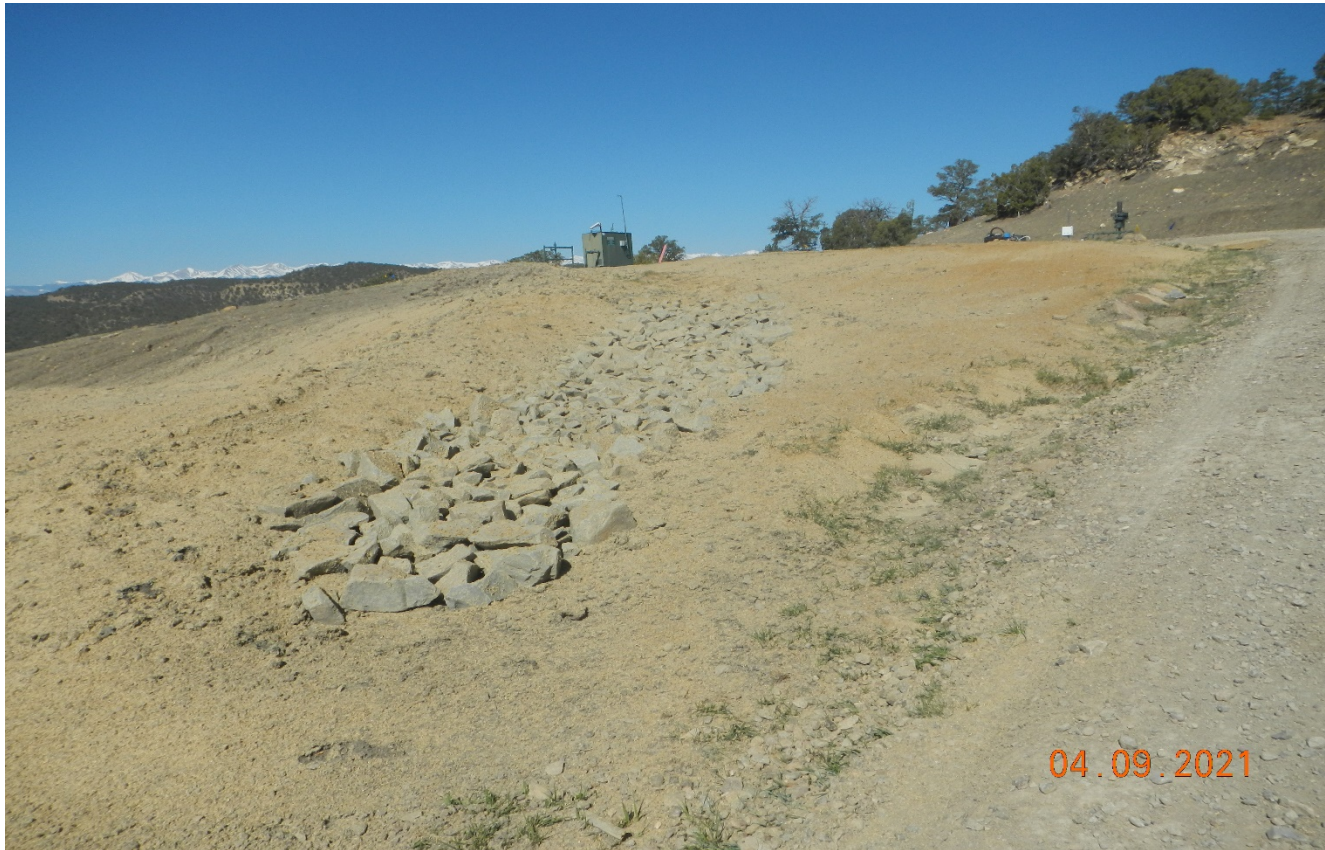
Photo 2. A portion of the fill slope of the location was seeded and hydromulched.
