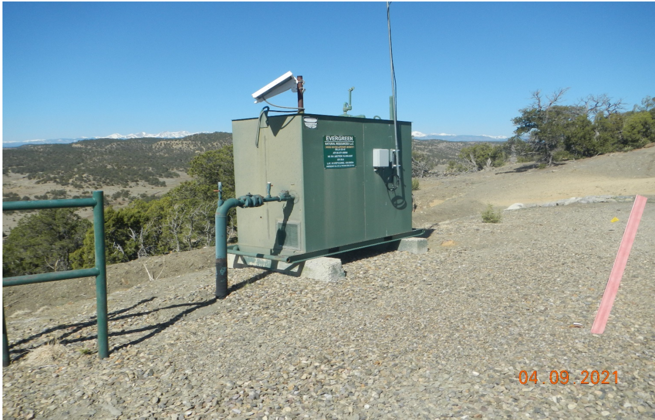
Photo 3. Well sign is posted at meter shed.
