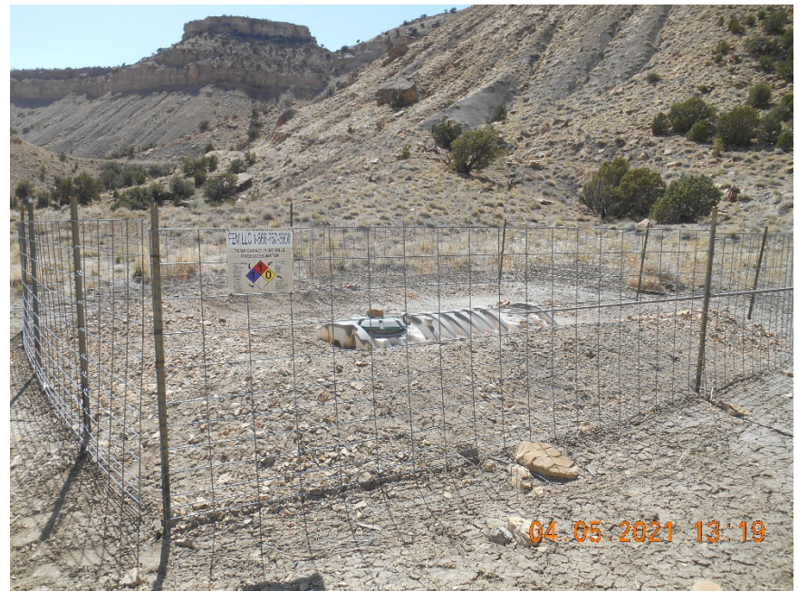
Dehydrator blowdown tank
