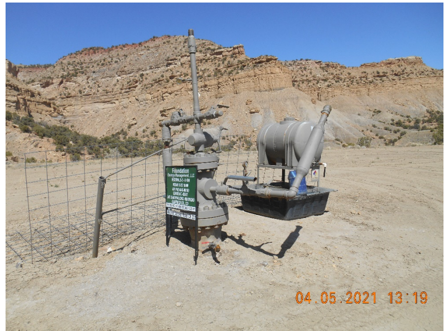
Wellhead with sign. Secondary containment of chemicals.
