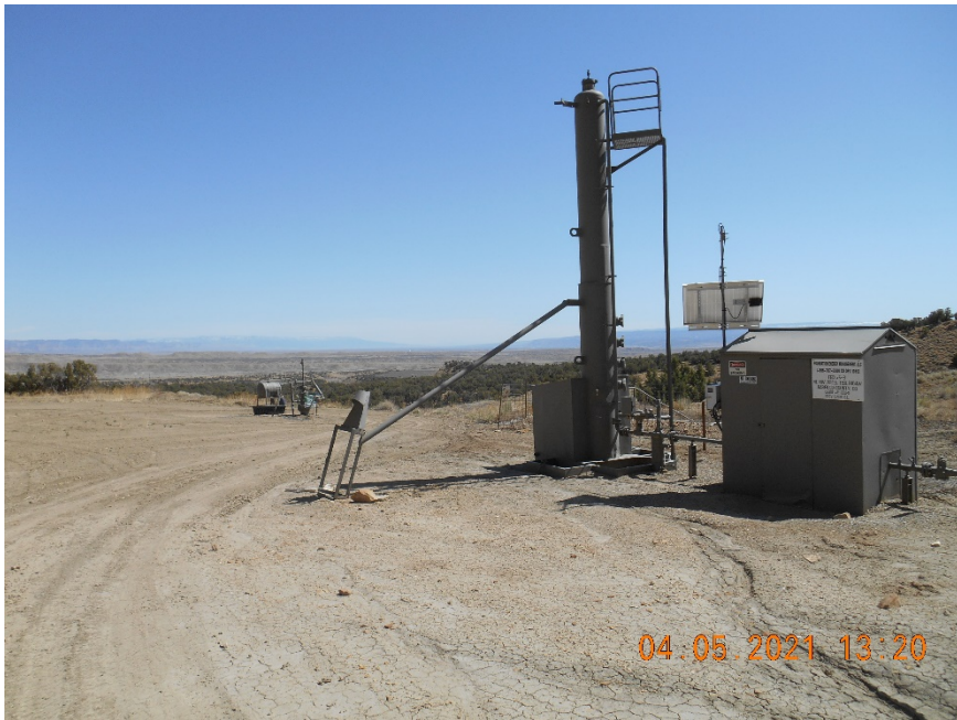
Dehydrator with blowdown tank, Meter housing and sign.
