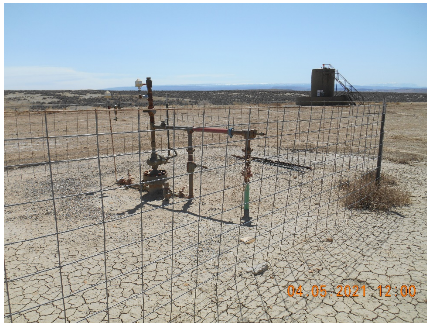
Wellhead with fencing.
