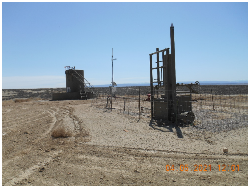
Separator with meter
