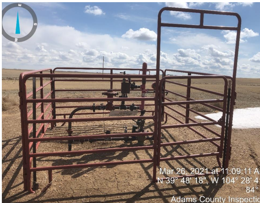
Photo #3 Well Head.
