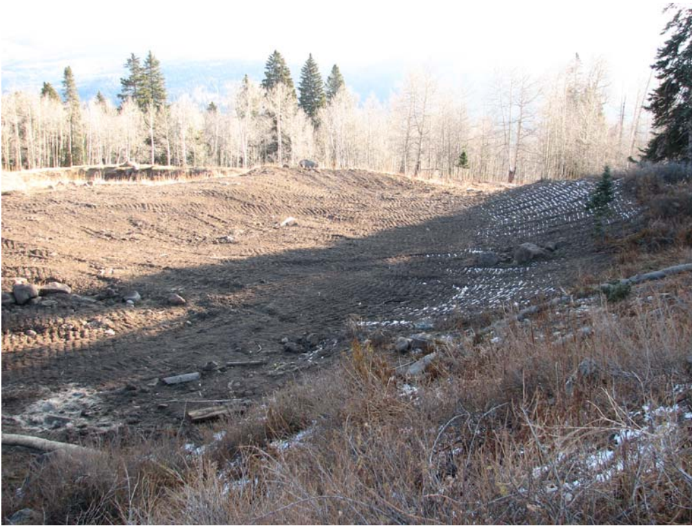
Overview of post remediation grading in the fall of 2008. Stormwater features had not been installed at this time.
