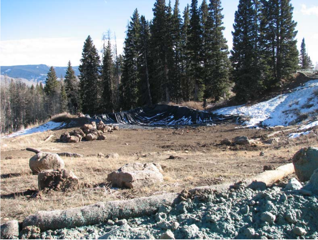
Typical view of impacted area in early Spring 2008. The lined area is the historic Sun Oil Company drilling mud pit and the target of 2008 remedial activities. The liner was installed as a component of the 2007 winterization effort.
