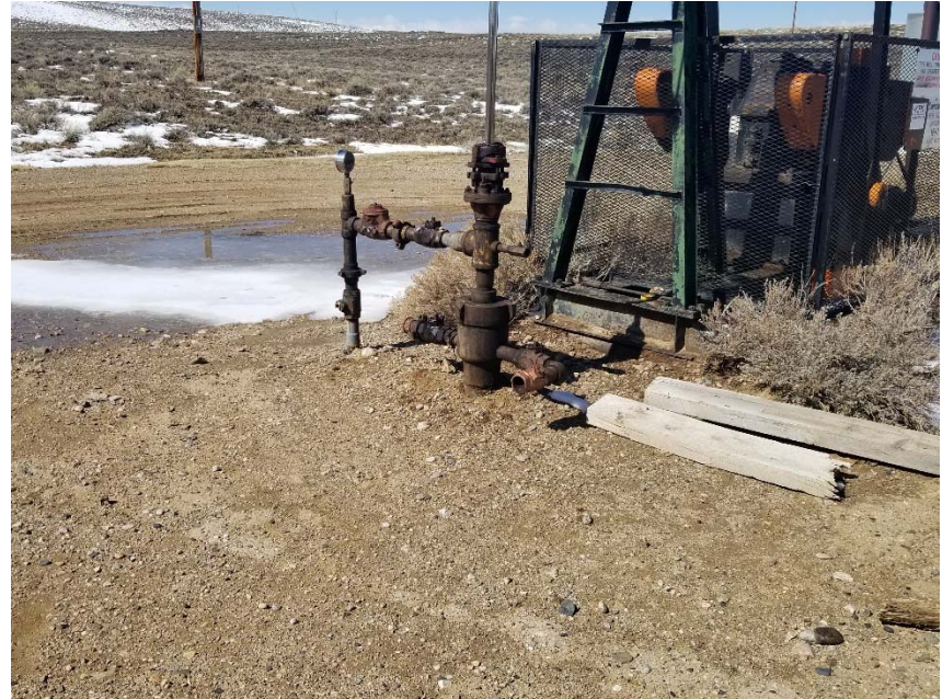
Photo 2. No bradenhead access apparent.
