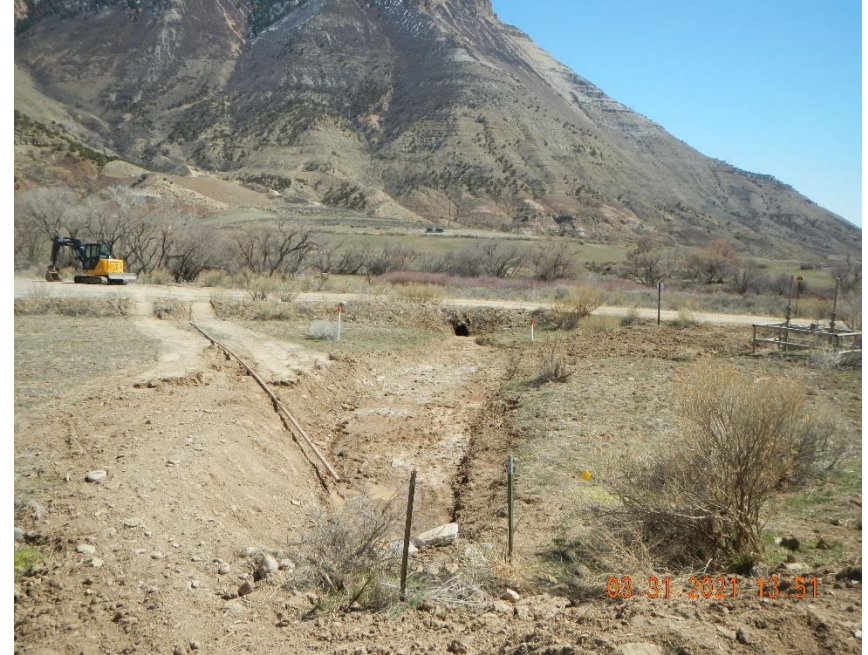
Tubing being used to clean out clean out culvert, unsure if it is the unused tubing form previous inspection.
