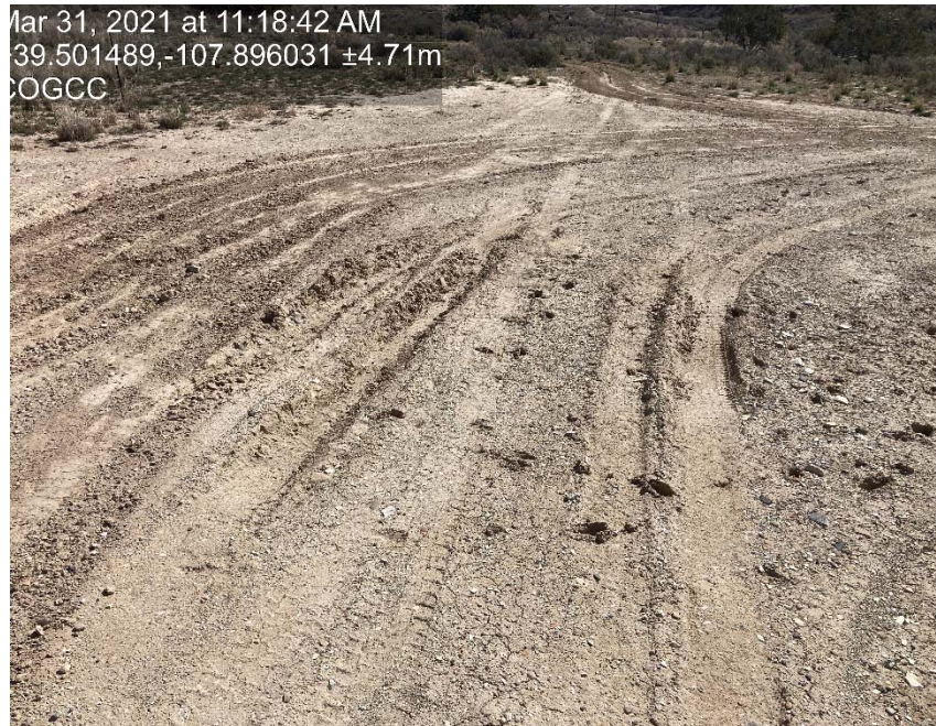
Lack of stabilization/compaction
