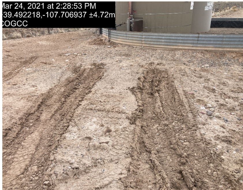
Lack of stabilization/compaction
