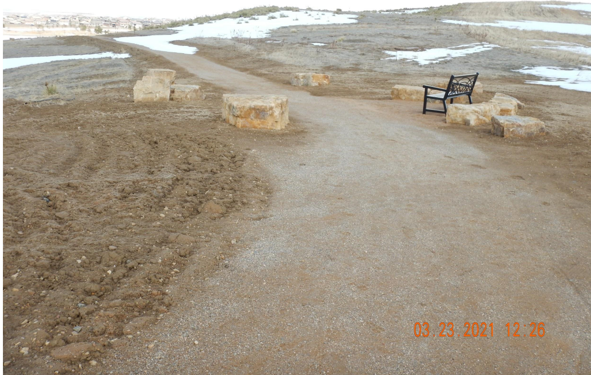
Photo 5. Photo taken from the well/tank battery location, facing North. Photo illustrates an open space path under construction.
