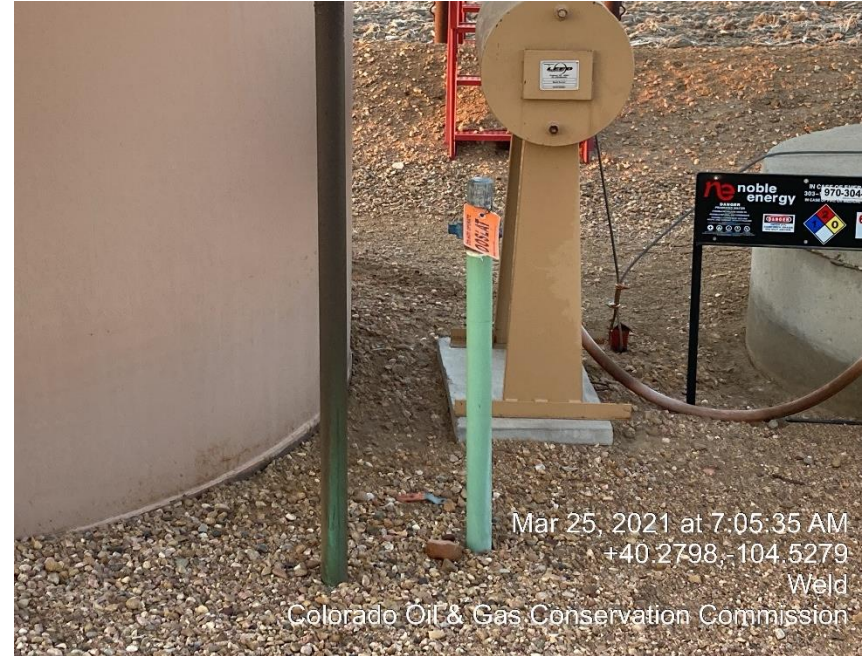
Photo #2 Marked Riser
