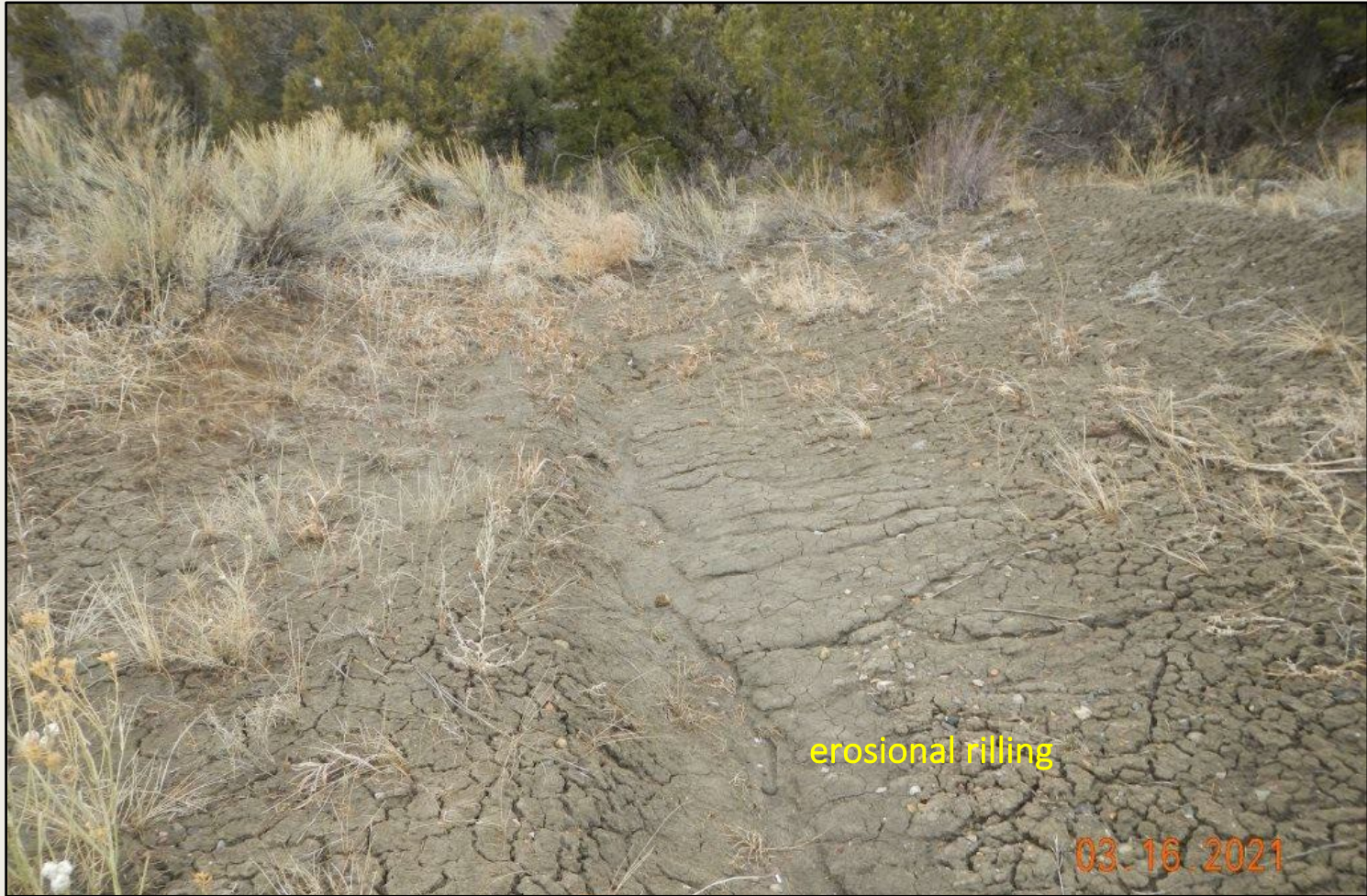
Photo 4. View of erosional rilling within the northwestern diversion channel facing downslope.
