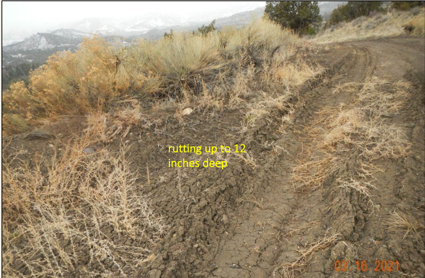
Photo 2. View of rutting along the access road up to 12 inches deep.
