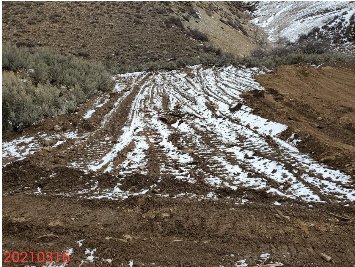
Photo 1: Photo taken from the northwest end of the Location, facing east. Photos 1-3 provide an overview of the Location from east, southeast, to south. Final reclamation work was in process at time of inspection.
