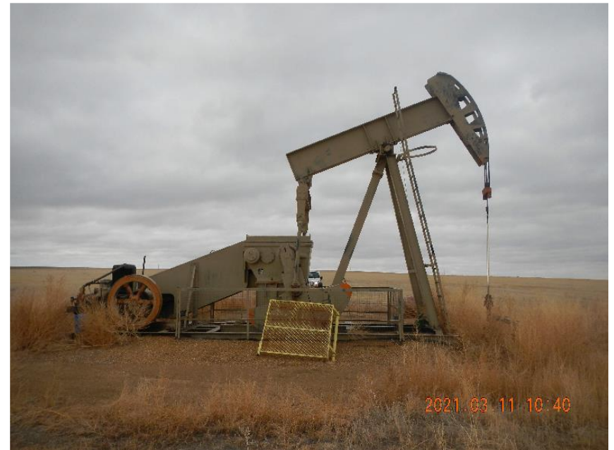
Photo 2: Additional view of pumping unit with removed guard visible.
