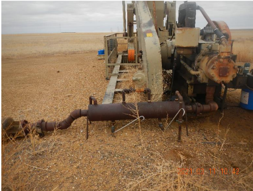
Photo 5: Knock out vessel at well.
