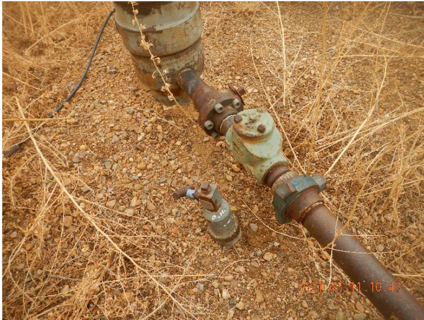
Photo 9: Braden head plumbed to surface.
