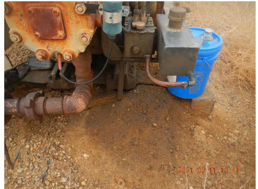
Photo 4: Impacted soil under and around prime mover.
