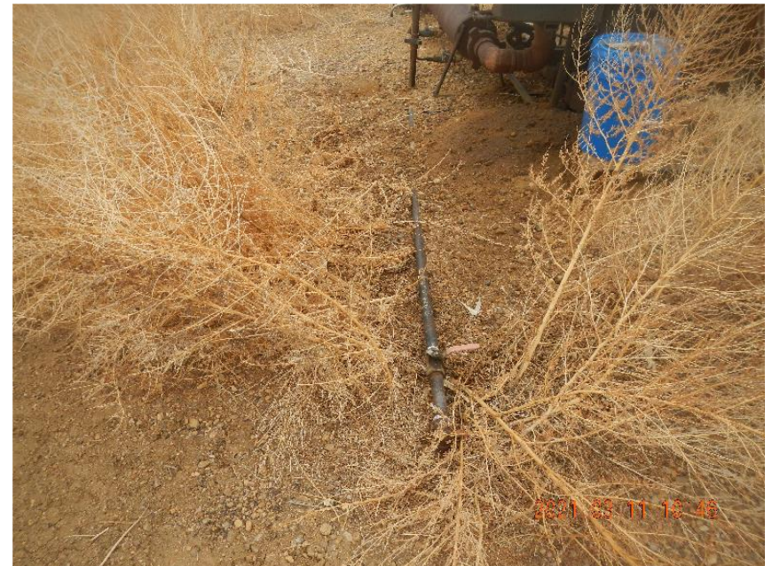
Photo 10: Supply gas line at well site.
