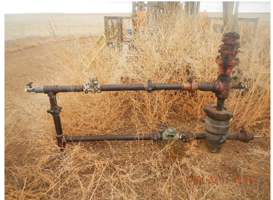
Photo 8: View of wellhead and tree.
