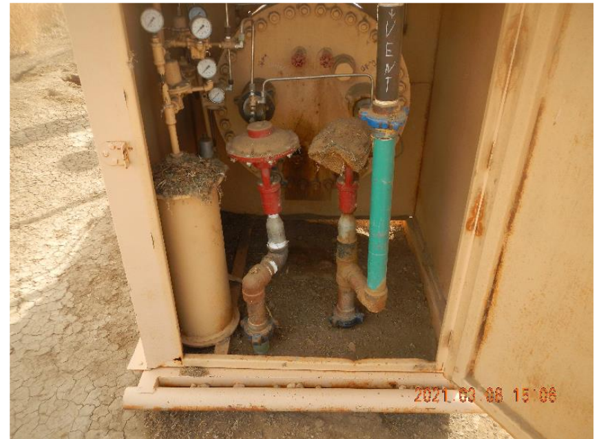
Photo 6: View of connected flowlines inside separator housing.
