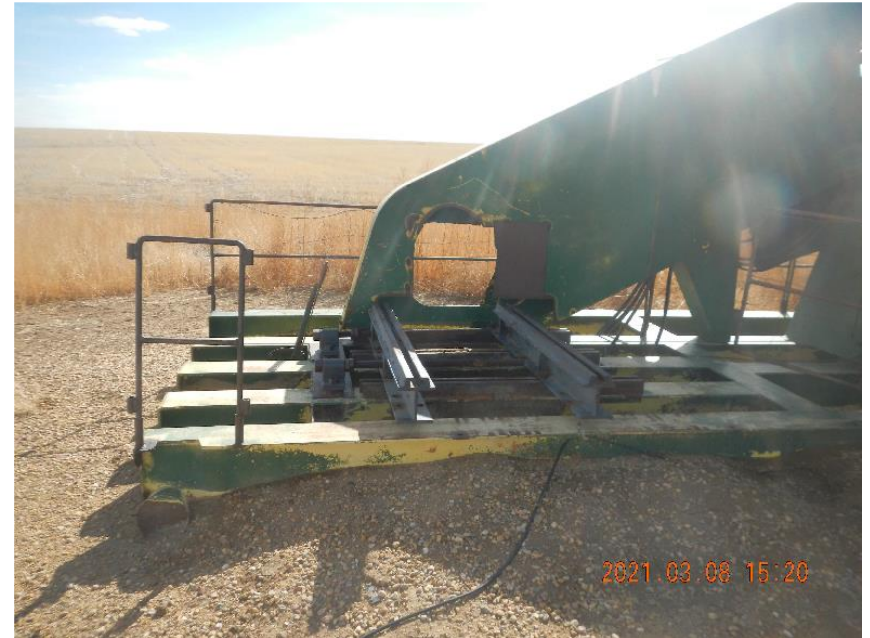
Photo 12: Pumping units prime mover has been removed.
