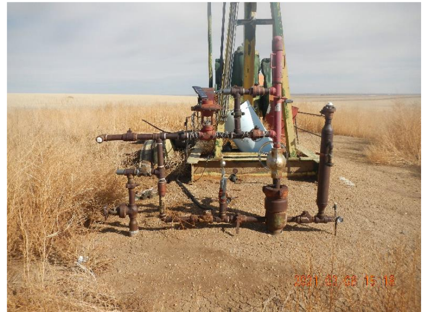
Photo 8: View of wellhead.
