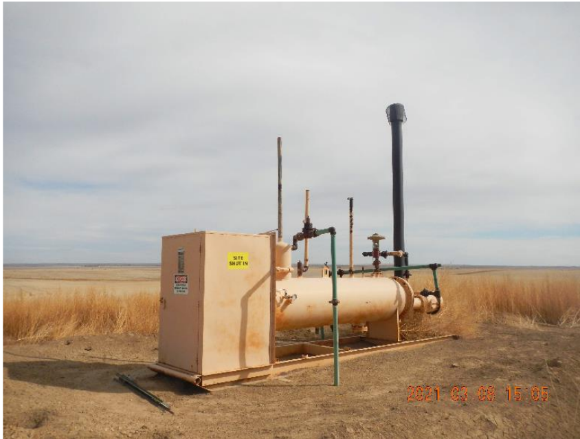
Photo 5: Horizontal heated separator.
