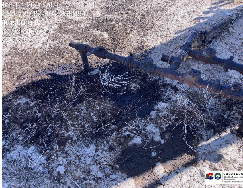
Pic 5 mechanical issue / stained soil
