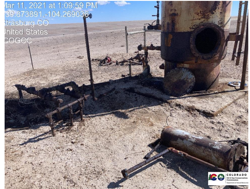
Pic 4 unused equipment / stained soil / mechanical issue
