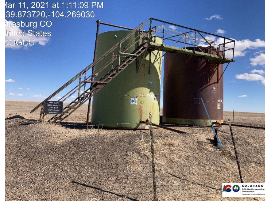
Pic 6 mechanical issue / stained soil
