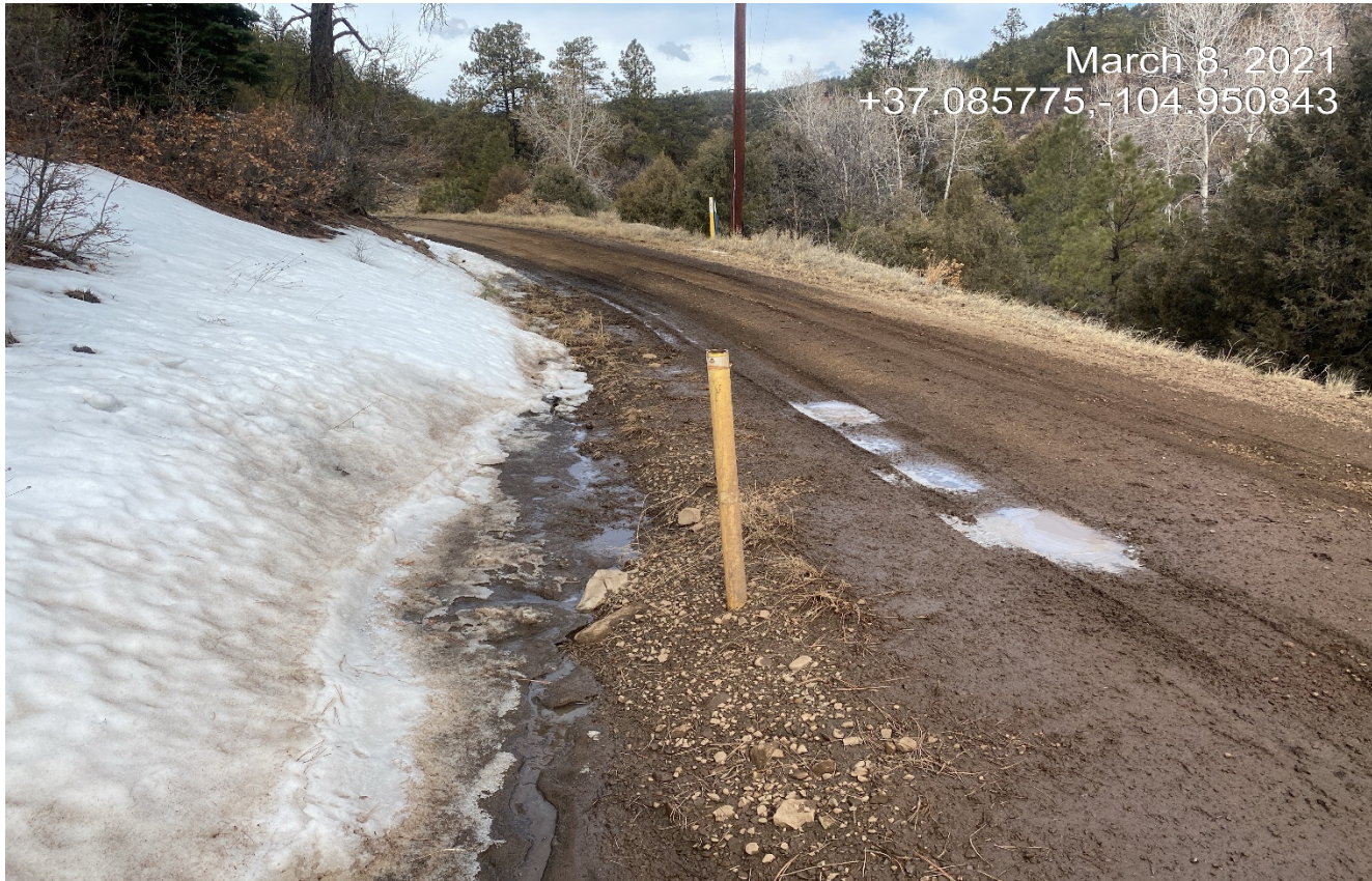
Photo 1. This culvert along the main road is filled in with sediment.
