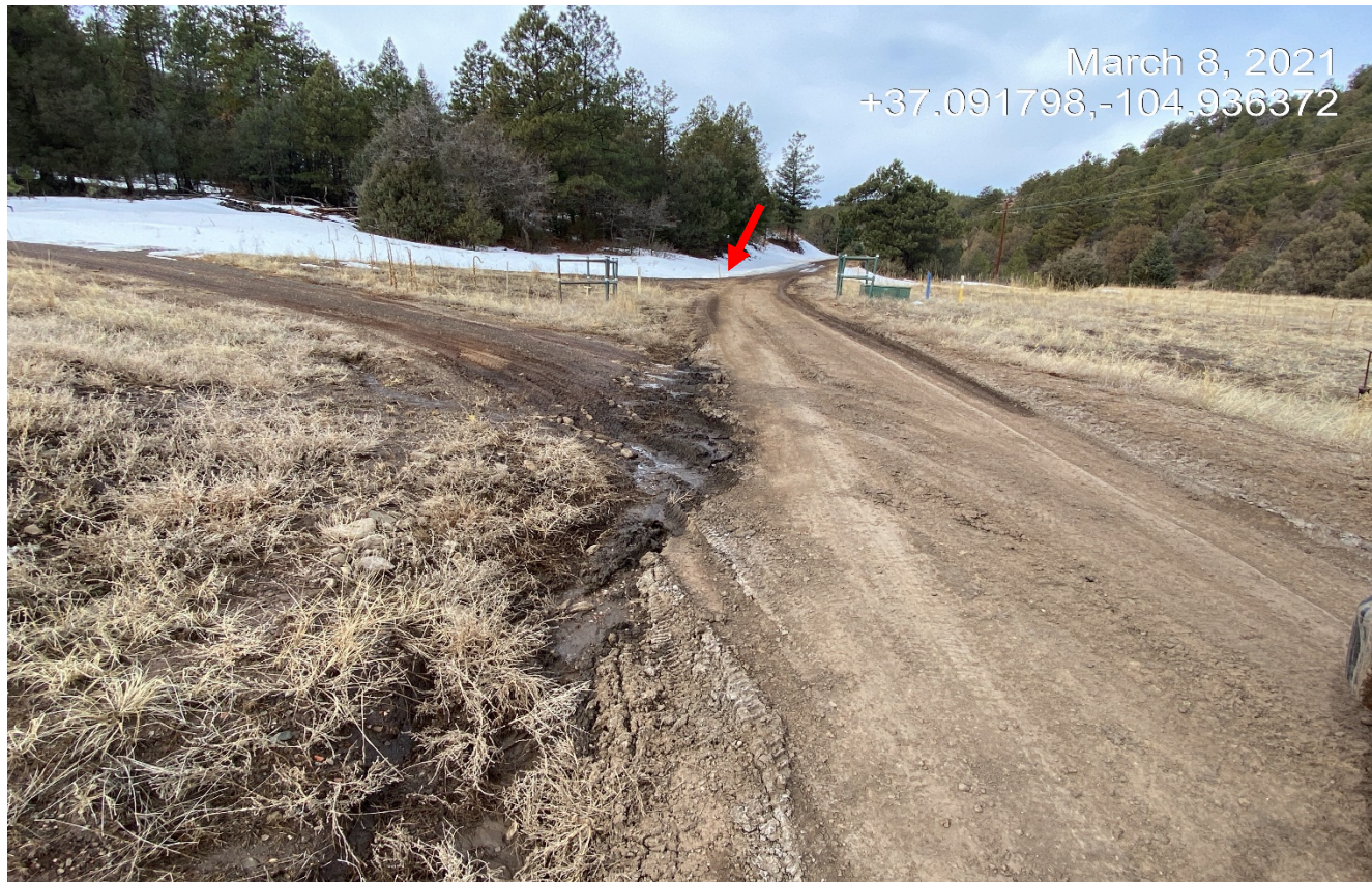
Photo 2. There is a plugged culvert along the main road (red arrow) causing stormwater to flow down the road. Lat/Long:37.09178,-104.93688. Previous corrective action was not performed.
