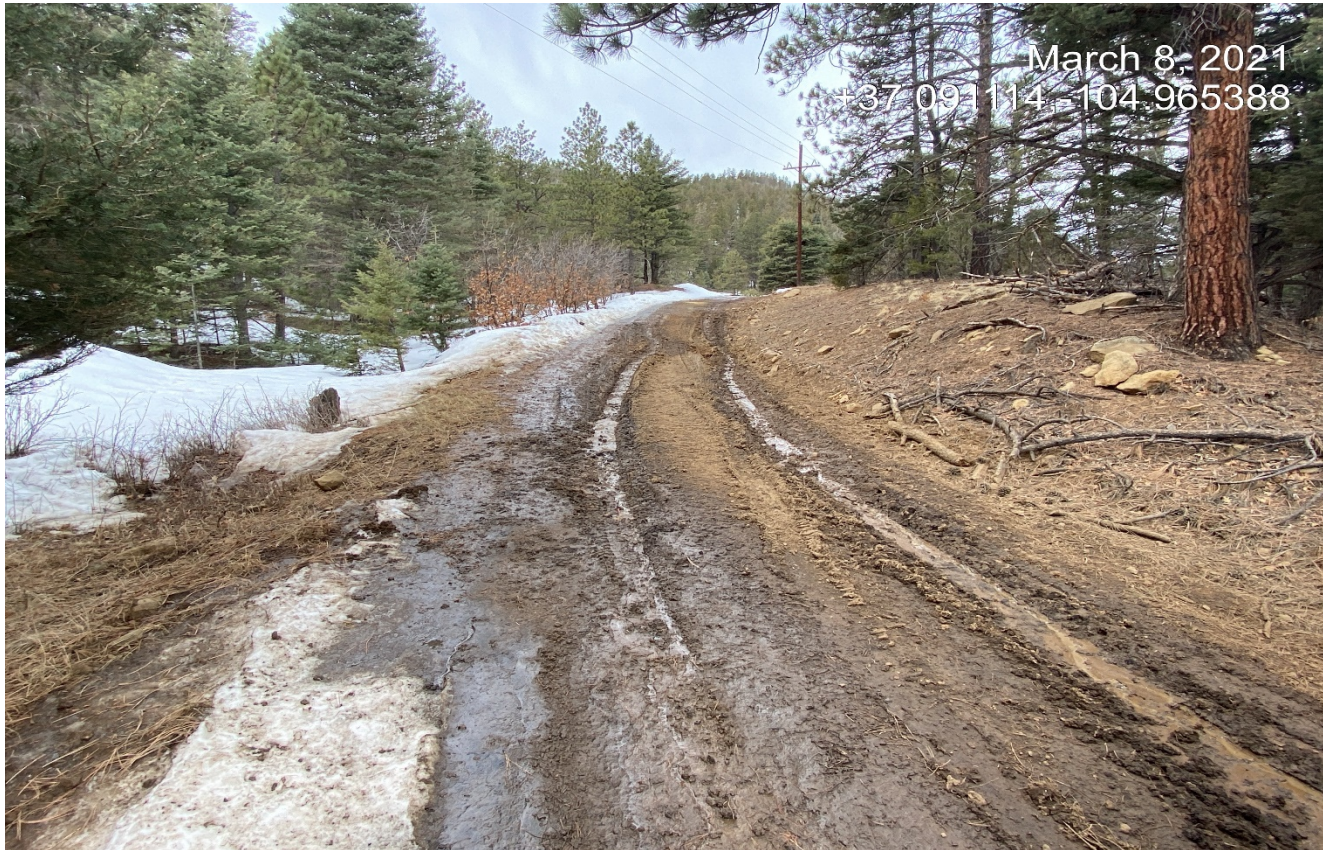
Photo 3. Vehicle rutting is occurring along the main road. Grading the road is not sufficient. BMP's need to be installed to prevent vehicle rutting.
