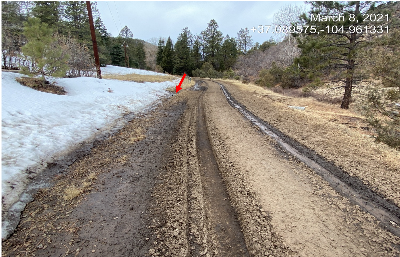
Photo 2. Stormwater is not directed toward the culvert (at red arrow) causing stormwater to flow on the road. Areas of rutting need to be stabilized with gravel and compaction.
