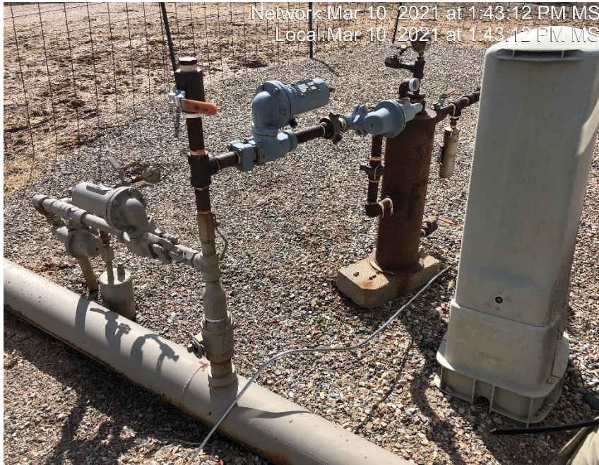
Photo #3111 Domestic tap off of sales line
