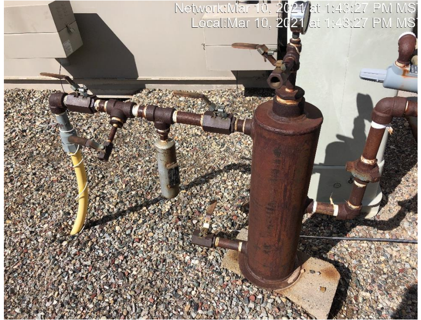
Photo #3113 Fluid knock out
