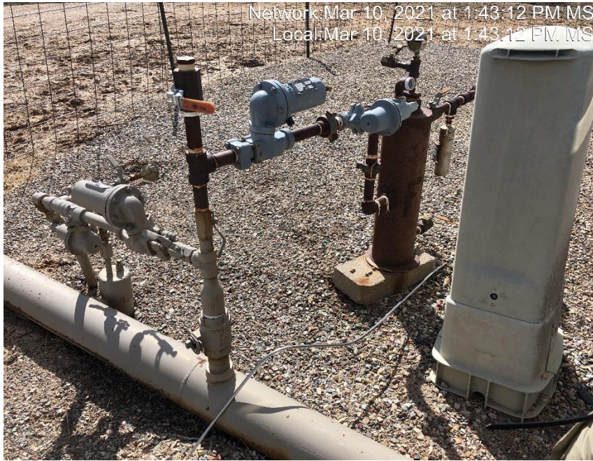
Photo #3111 Domestic tap off of sales line
