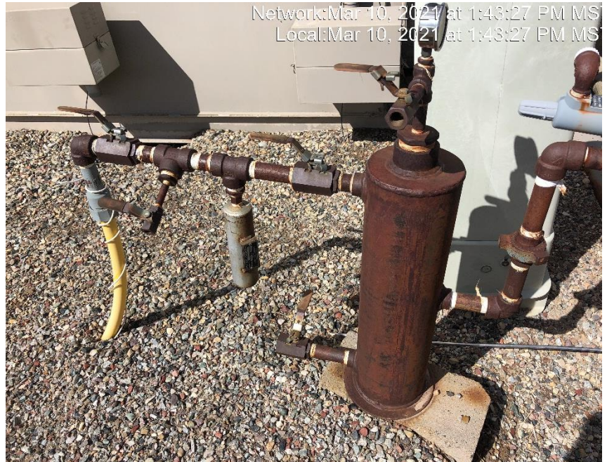
Photo #3113 Fluid knock out
