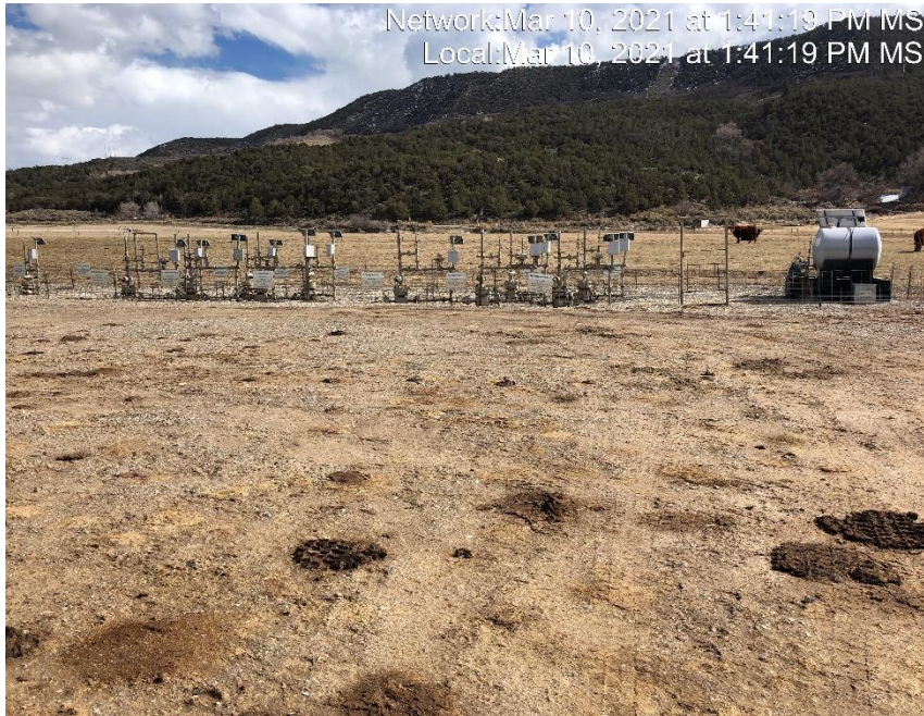
Photo #3109 from entrance to Wellheads
