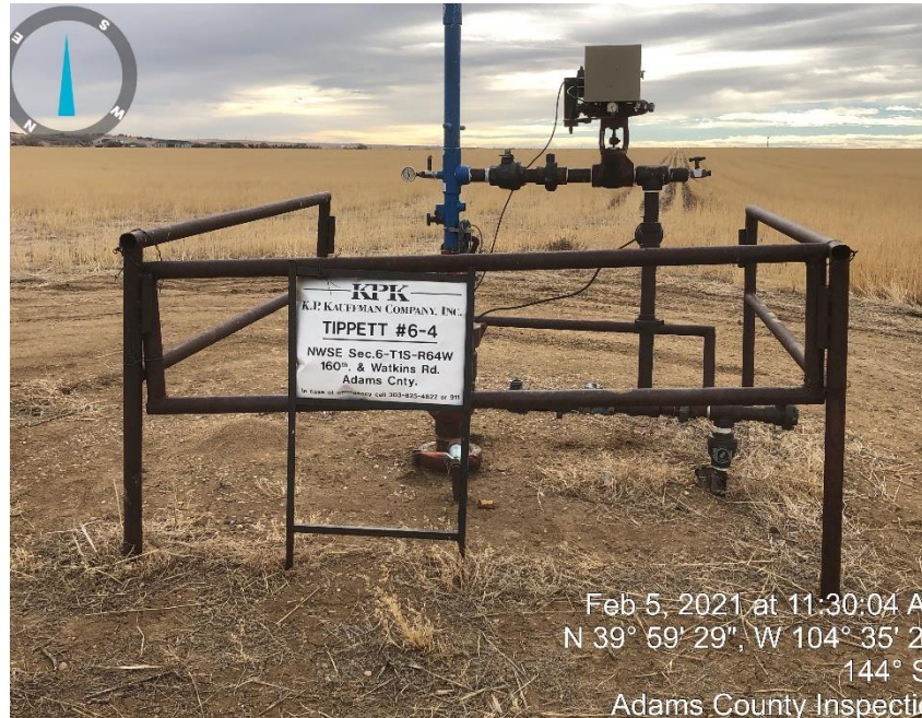
Photo #3 Well Head.
