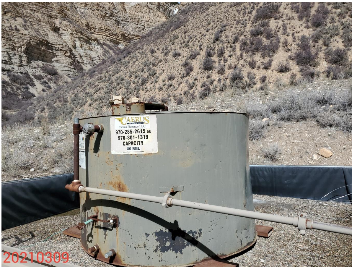
Photo 6: Photo of tank on the northwest end of the Location, and signage.
