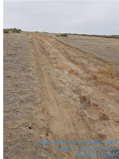
2. Erosion on access
