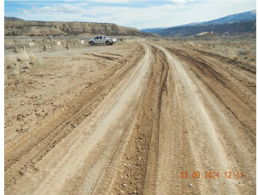
Rutted access road looking east.
