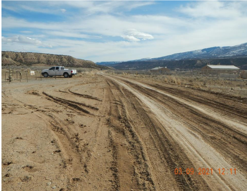
Ruts on location and access road.
