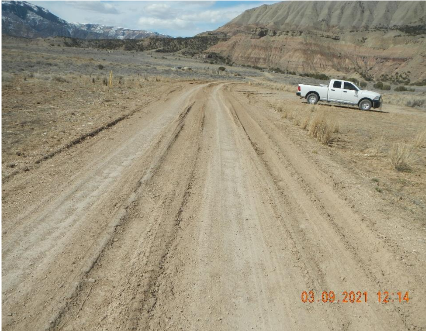
Rutted access road looking west.
