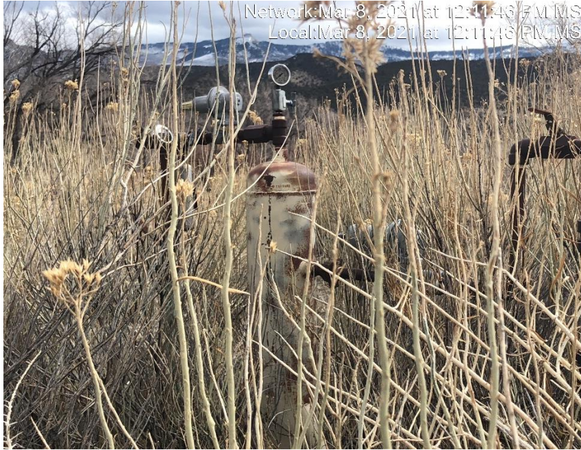
Photo #3092 Fluid knock out and little joe regulator.
