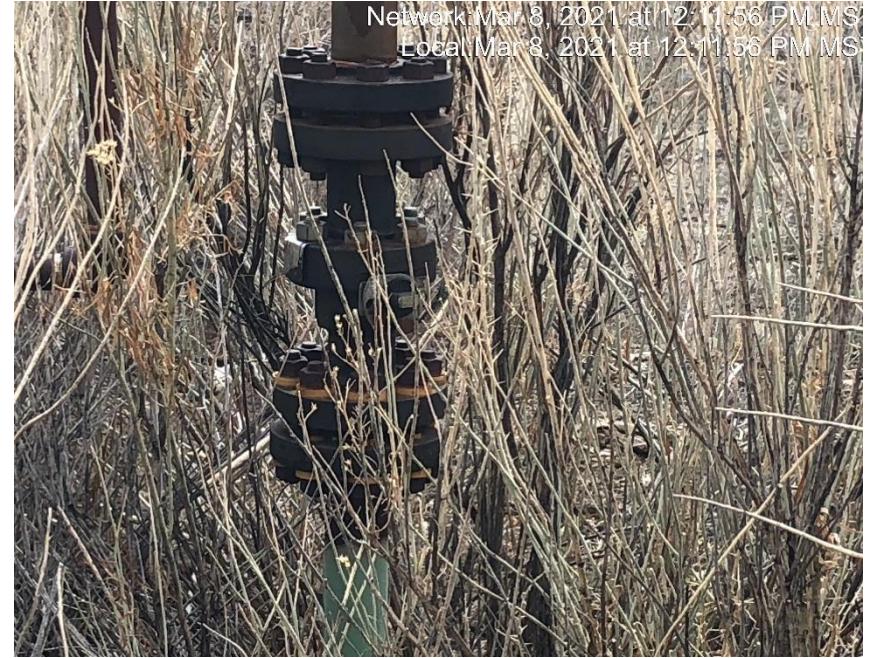
Photo #3093 Isolation valve closed.
