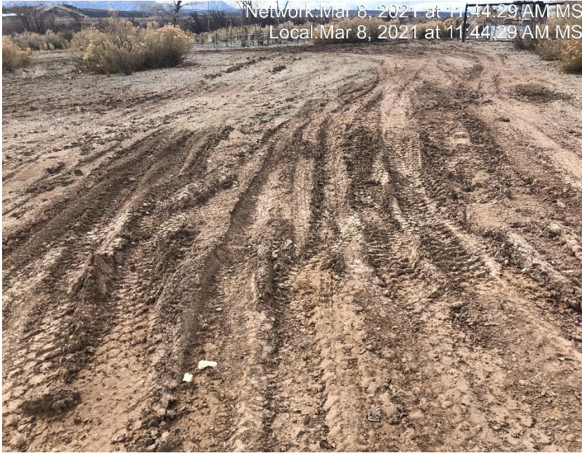
Photo #3086 Rutting present on location due to lack of stabilization.
