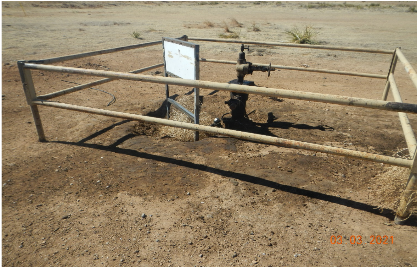
Photo 7. There is oil stained soil around the wellhead.
